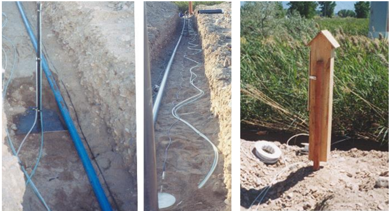
Figure F10. Settlement manometer standpoint (left). Plastic tubing (center). Housing box with measuring staff inside (right). Note inclinometer casing and pressure cell have also been installed at this site.
