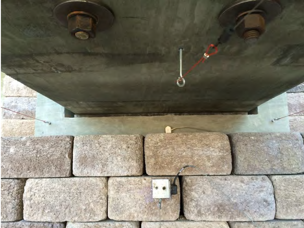
Figure A2.19 Accelerometers on the facing block and bridge seat.
