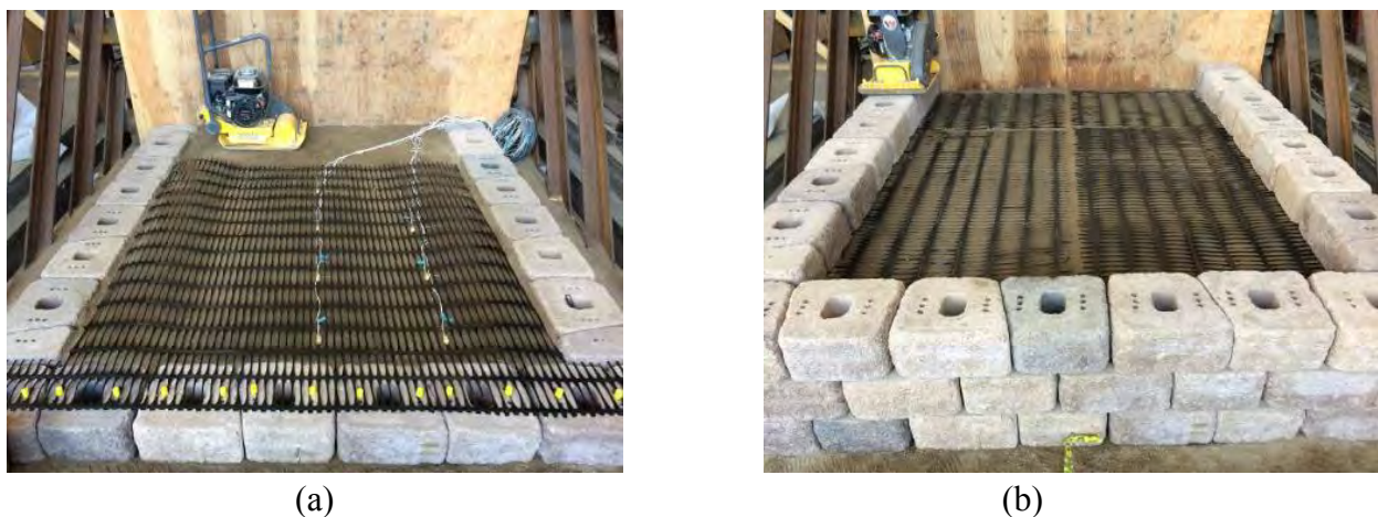
Figure 3.28 Construction of MSE bridge abutment: (a) longitudinal reinforcement layer; (b) transverse reinforcement layer.
