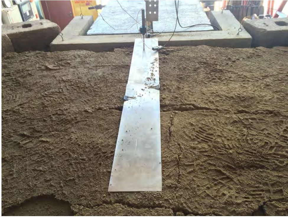
Figure A2.37 Crack after all shaking motions for Test 2.
