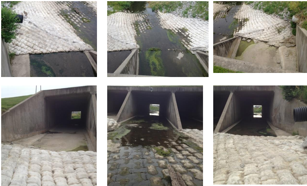
Figure 5A. Views of the mat-covered fillets as applied at the inlet of a 15'-18"-15" x 12 RCB on Hwy 1 W, Iowa City. Note: there is a slight difference in the fillet geometry compared to the specifications provided in Appendix A. The geometry has been updated based on observations during the monitoring of the implemented design.
