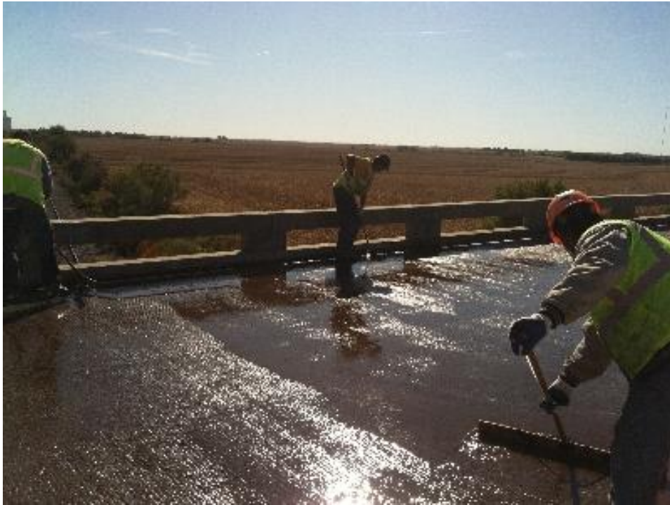
Figure 2.1. Typical placement of resin for multiple-layer concrete overlay (Courtesy: KwikBond Polymers). Resin is applied followed by an aggregate broadcast.
