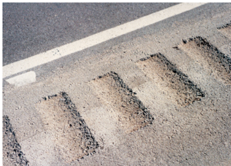
Milled Rumble Strips
