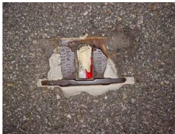
Figure 8. RSPM with broken casting and lens
