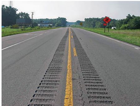
a) Rumble strips
