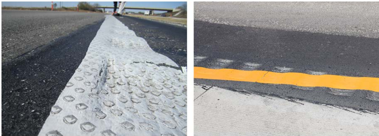
Figure 14. End of project condition for trailing edge-line markings
