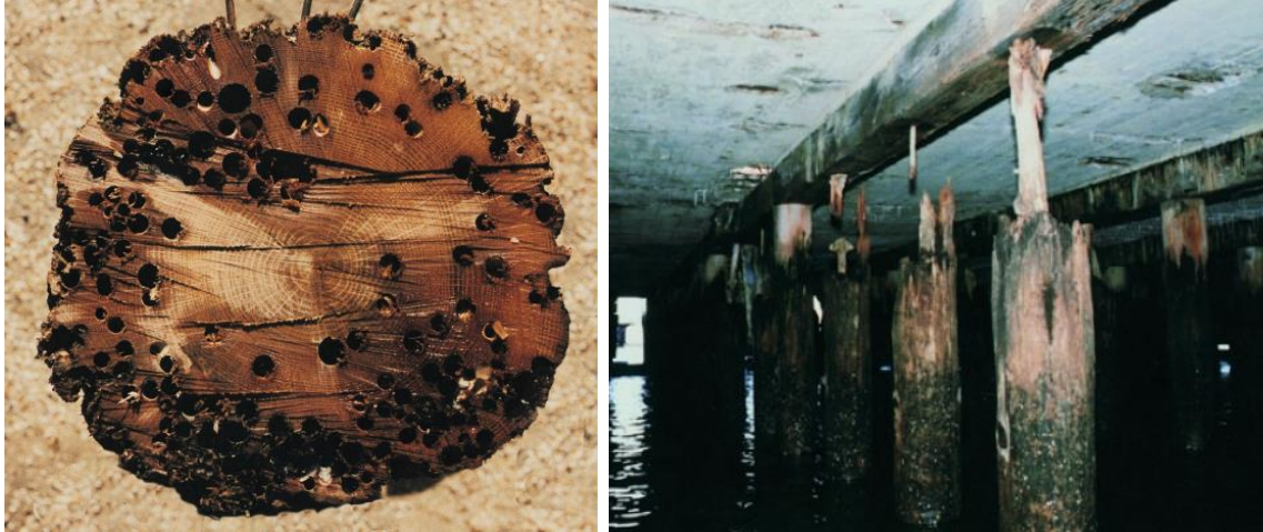
Figure 1: Tunneling in a timber pile caused by Teredo and Bankia (left), untreated timber piles attacked by Limnoria (right) [16]
