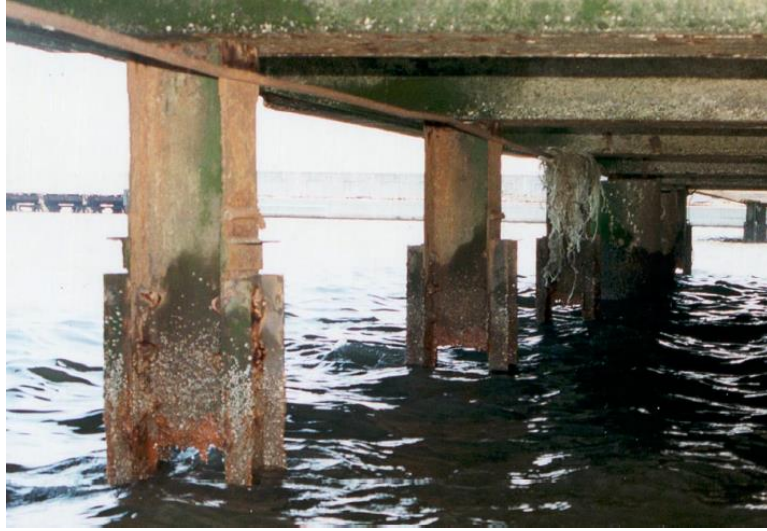
Figure 2: An example of corroded steel H pile supporting a harbor pier [16]
