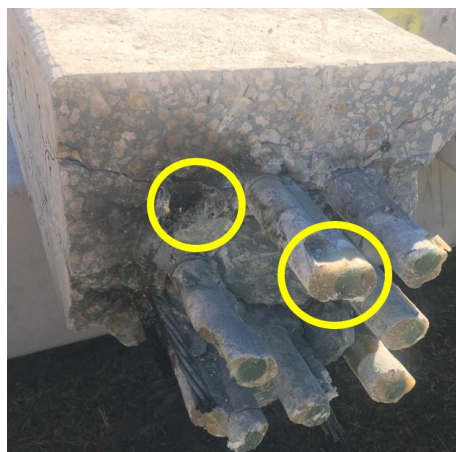
Figure 128: The oversized slanted holes
