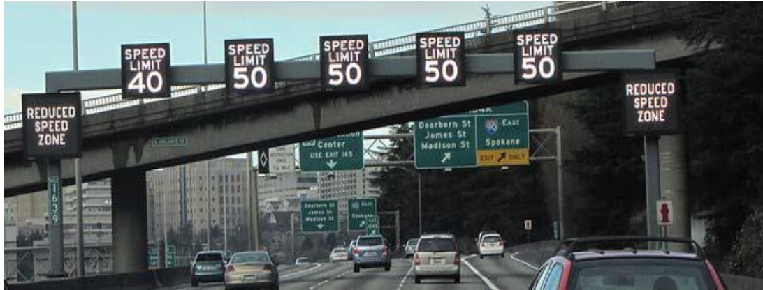
Figure 2.2 Overhead displays used along IH 5
