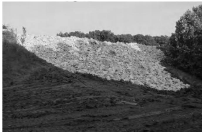
Figure 2-27 Typical soil substitution method (Reprinted from “Slope Maintenance and Slide Restoration Reference Manual” by Collin et al., by permission of James Collin, Year of first publication: 2008)
