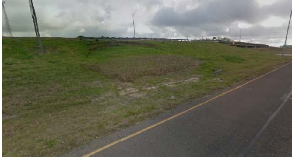
Figure 5-9 Slope failure on South US 69 at Chinn Lane
