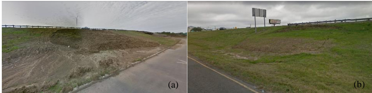
Figure 5-4 Slope failures in Beaumont, TX, after Hurricane Harvey: (a) North US 69 at Fannet Road Junction and (b) South US 69 at Lower Neches Valley Authority
