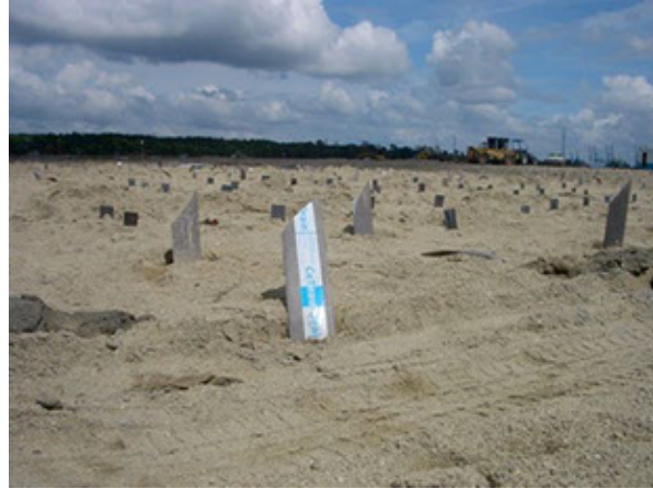
Figure 2-44 Wick drain installation (Reprinted from “Prefabricated Vertical Drains” by CeTeau, by permission of de Zwart, Year of first publication: 2017)
