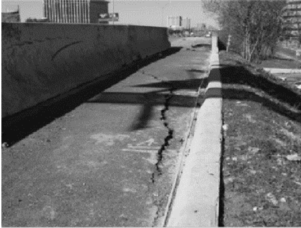
Figure 5-12 Crack and surficial movement of the slope (Hossain et al. 2017)
