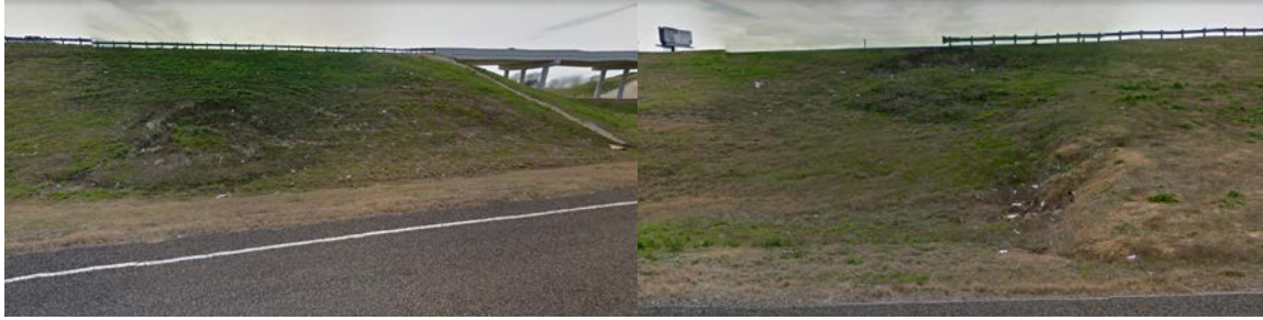
Figure 5-18 Failure of fill slope on US Highway 287 North near the St. Paul overpass in Midlothian
