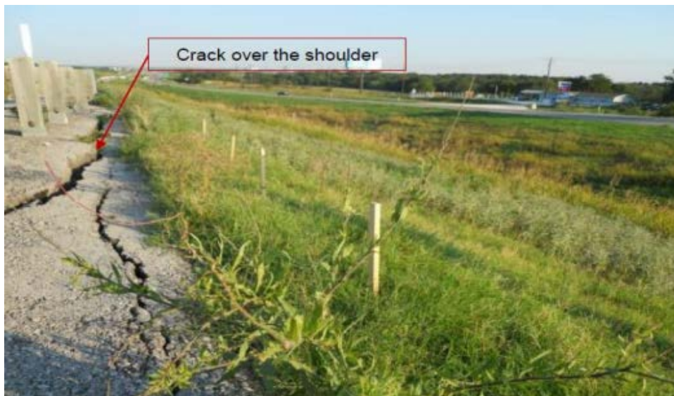
Figure 5-17 Crack and surficial movement of slope (Tamrakar 2015)
