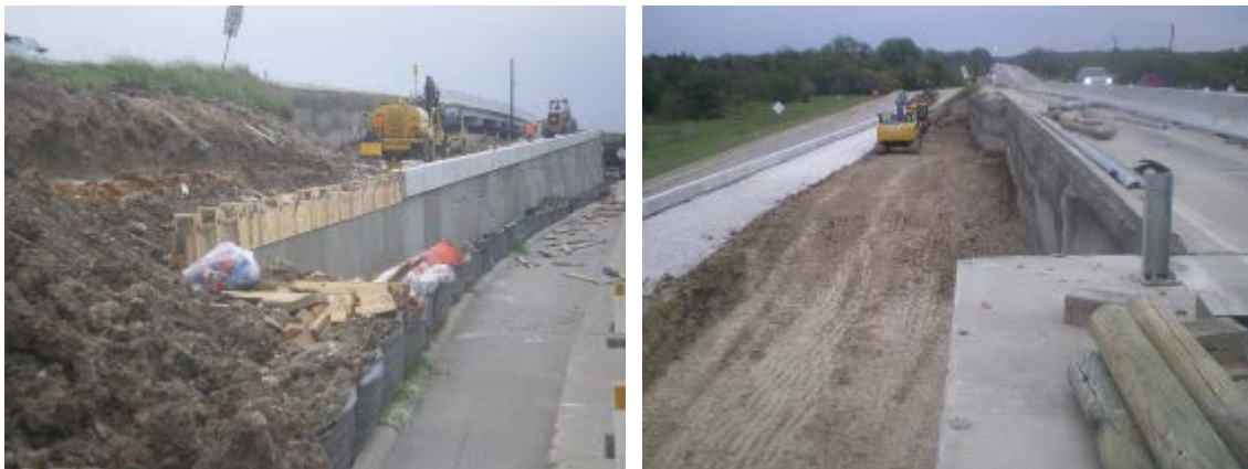
Figure 5-24 Installation of concrete retaining wall, backfilling and compaction (photo courtesy of Nicasio Lozano)
