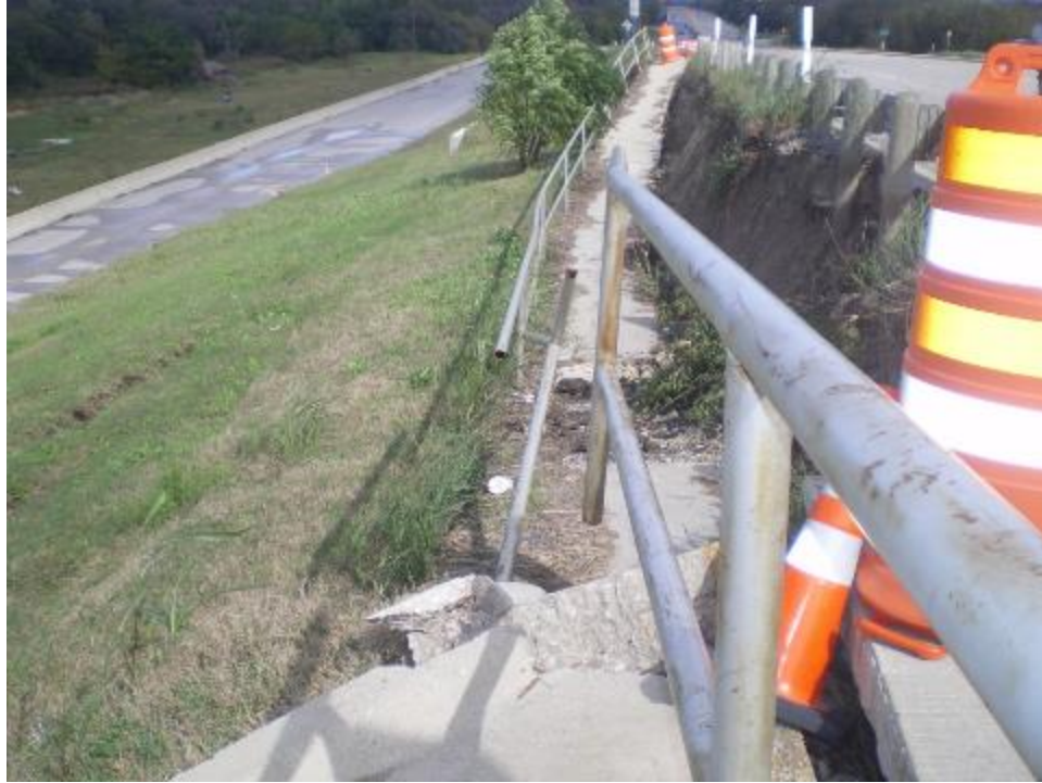
Figure 5-21 Slope failure on the West Texas Loop 12 (photo courtesy of Nicasio Lozano)
