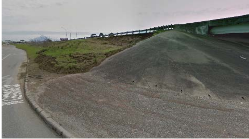
Figure 5-6 Slope failure on North US 69 at TX-93 Spur
