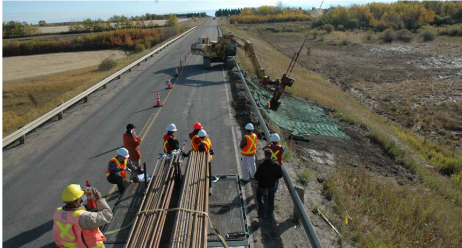
Figure 2-11 Use of SNL method in urban Access Road 172 Slope Repair Project (Smith et al. 2009)
