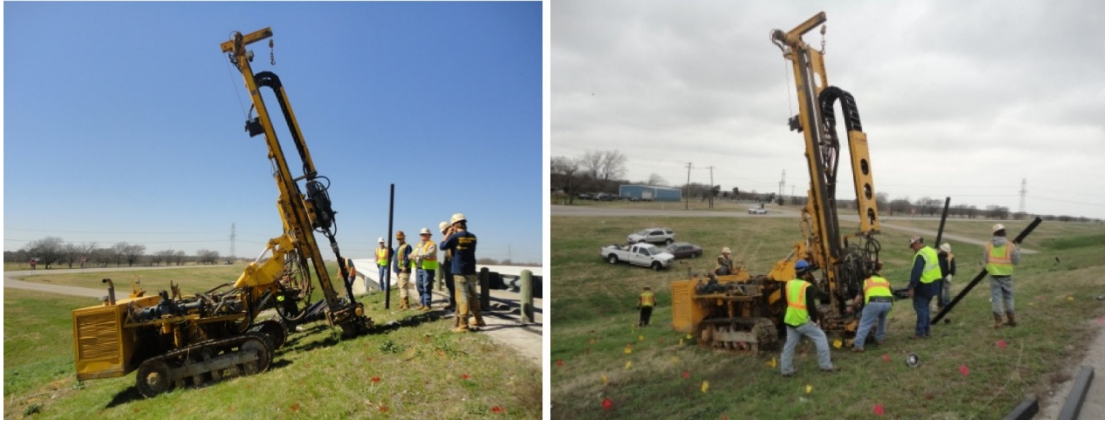
Figure 2-14 Installation of recycled plastic pins on U.S. Highway 287 near the St. Paul overpass in Midlothian, Texas (Khan et al. 2017)
