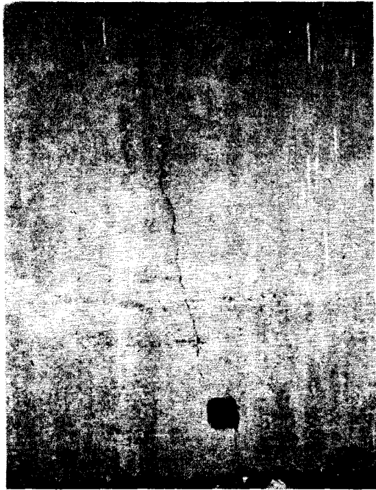
Figure 5. Minor cracking in abutment caused by differential settlement.
