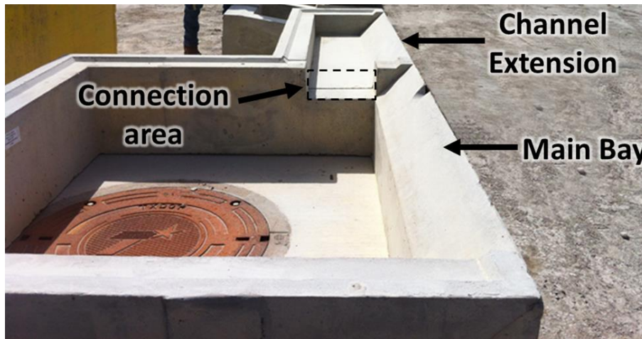
Figure 3: Upper inlet basin of TxDOT PCO 10-ft inlet. Manhole and concrete floor are of separate component on which the upper inlet is stacked (photograph courtesy of TxDOT).
