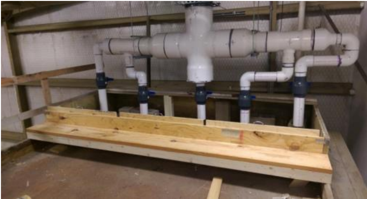
Figure 18: Inlet pipe manifold with valves, and headbox.
