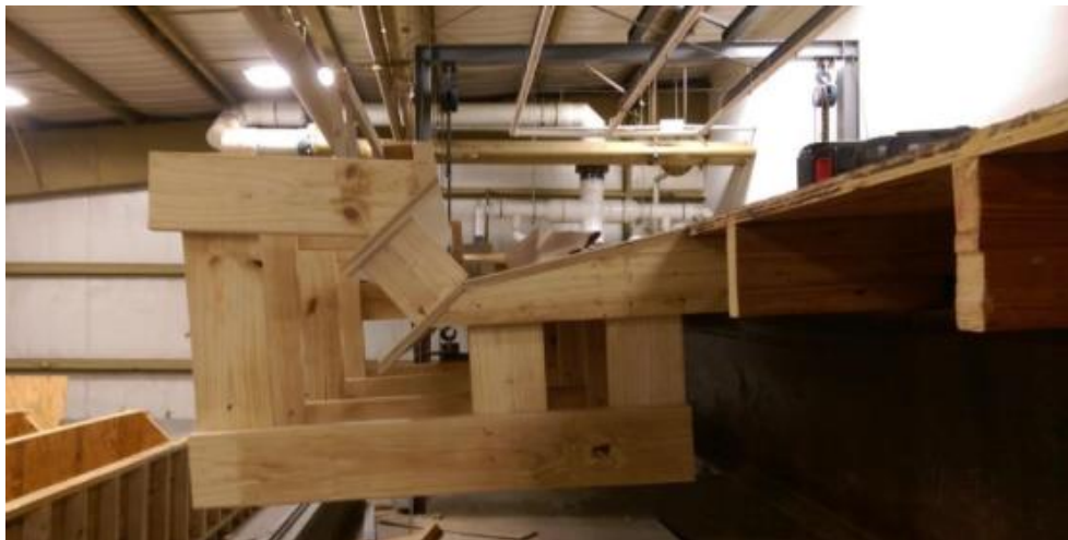
Figure 20: Under construction – view from downstream of the 2x6 inch wood framework for conventional 15 ft inlet.
