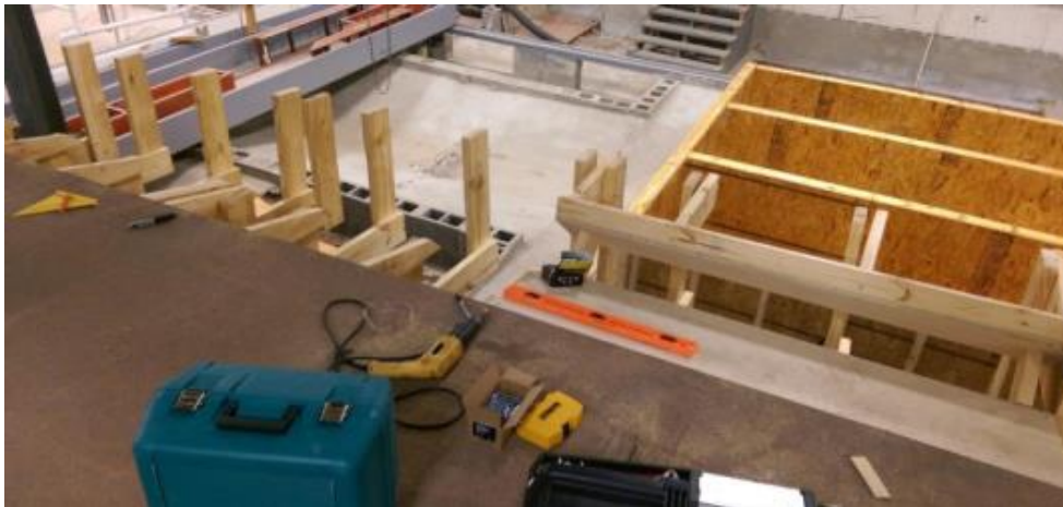
Figure 19: Under construction – wood framework of 2x6 inch studs for conventional depressed inlet.
