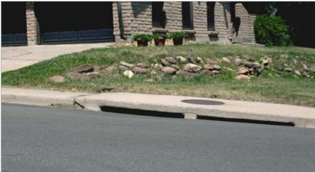
Figure 6: Curb inlet (depressed) with flush slab support (Denver Urban Storm Drainage Criteria Manual, V. 1, pg. ST-20).
