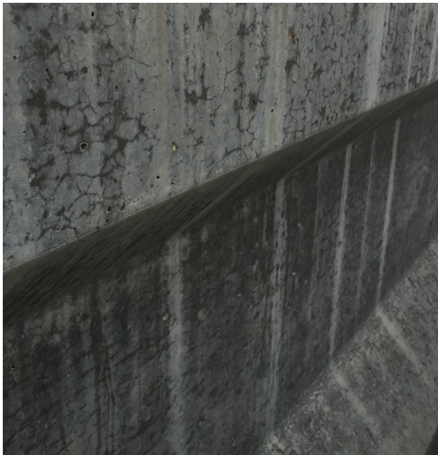
Figure 1: Micro-cracking focused on the top flange at a TxDOT producer precast plant
