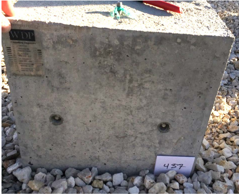
Figure 6-2: Example of Crack Rating = 1
