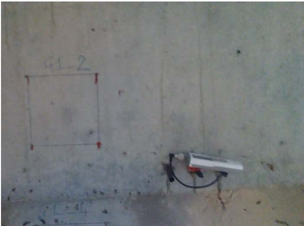
Figure 2-14: Overall photo of G1, an exterior uncracked girder, with corresponding humidity measurement probes and crack map G1-2
