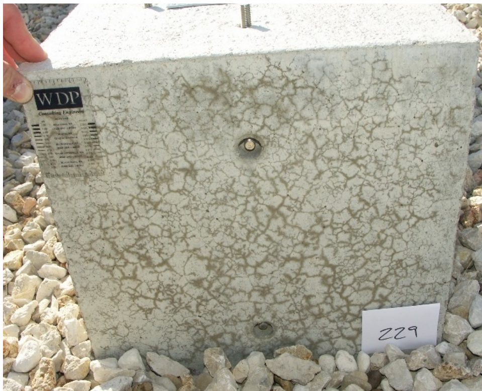
Figure 6-5: Example of Crack Rating = 4.5
