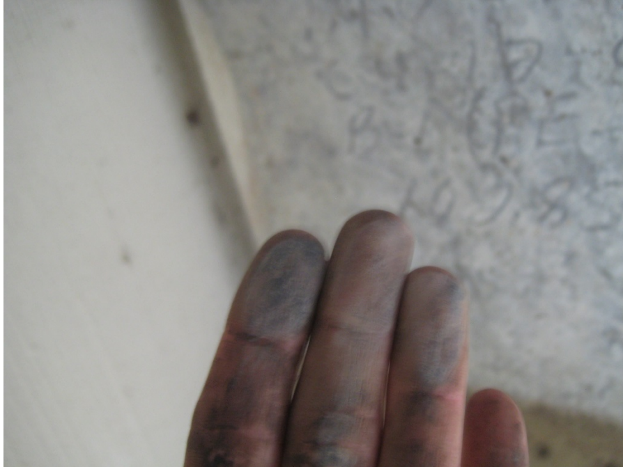
Figure 2-19: White powder on girders.
