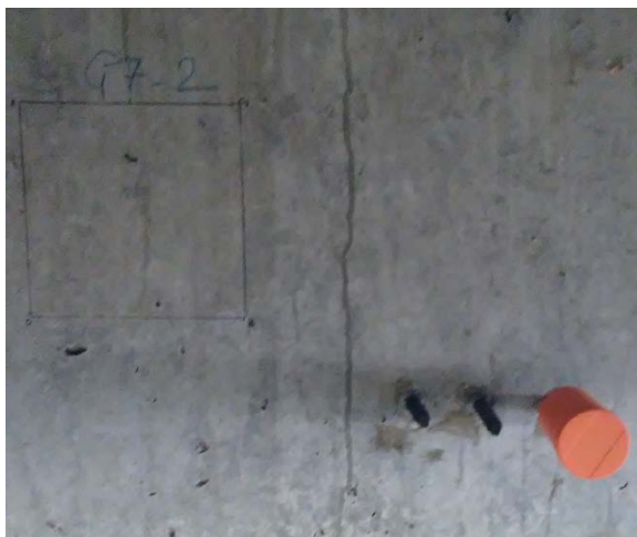
Figure 2-9: Overall photo of G7 with corresponding humidity measurement probes and crack map G7-2
