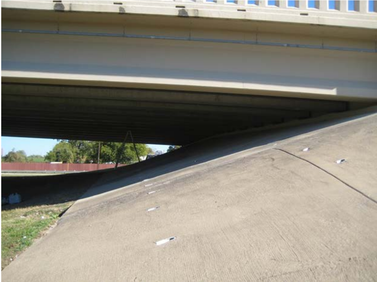
Figure 2-8: Overall view of bridge looking east; (exterior girder in this picture is labelled as G1)
