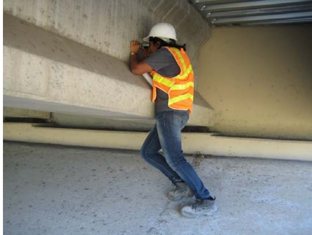
Figure 2-5: Savitha Srinivasan (graduate student working on associated TxDOT project 0-6922) recording crack widths and lengths at the Dallas site visit
