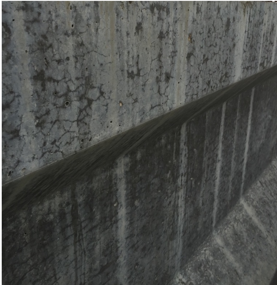
Figure 2-1: Micro-cracking focused on the top flange of a rejected precast girder
