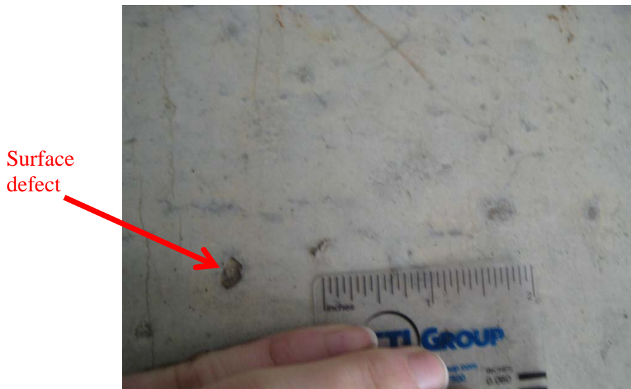
Figure 2-22: Similar surface defects observed in cracked flange at Texarkana
