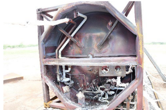
Figure 6. Post-Test Photograph of Piping Cabinet of Test Tank
