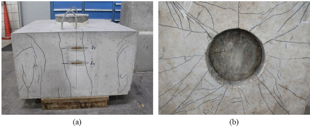
Figure A.110: Cracking on the (a) east side and (b) bottom of specimen S2-13
