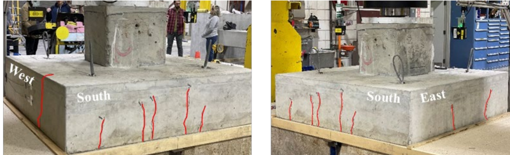
Figure B.45: Crack pattern at 350 kips for SC-1
