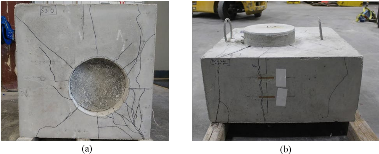
Figure A.204: Cracking after testing on (a) bottom and (b) cap of Specimen S3-10
