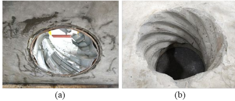
Figure 3.3: (a) Removal of corrugated pipe and (b) surface finish after removal of pipe and sandblasting
