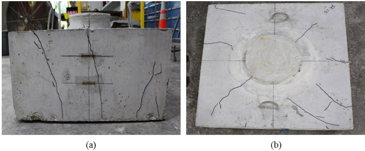
Figure A.118: Cracking on the (a) north side and (b) top of the cap
