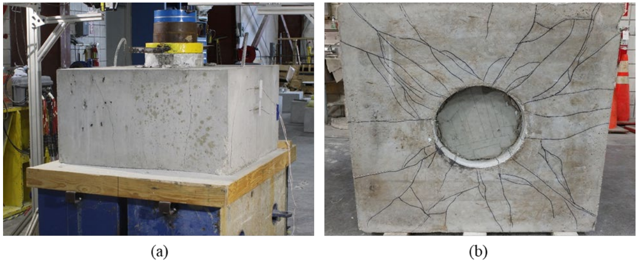
Figure A.138: Cracking on the (a) south side and (b) bottom of Specimen S2-20
