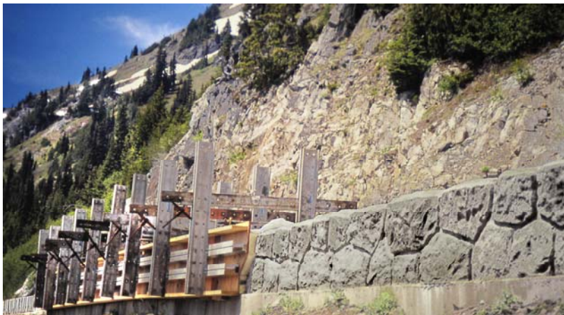
Forms remain in place at the left until the concrete achieves its initial set. At right, forms have been removed from an earlier pour. The insides of the forms are textured to give the concrete guardwall an appearance of stonework.
