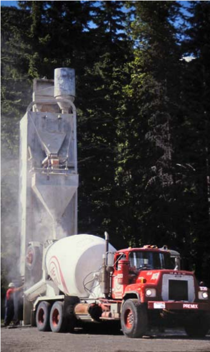
A portable batch plant erected on the project adds cement to a truck. Trucks left the supplier in Yakima loaded with sand, water, and gravel.
