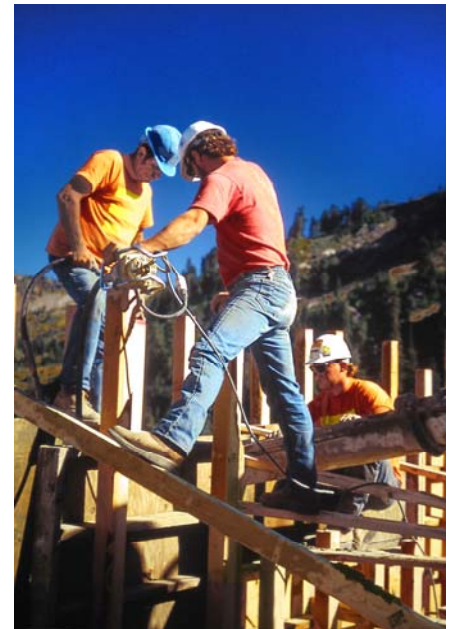
Laborers use a vibrator to consolidate the fluid concrete. This eliminates air bubbles and ensures sand and gravel are distributed evenly.
