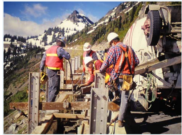
A truck delivers concrete to the guardwall forms. Sixty linear feet of forms are filled at a time.
