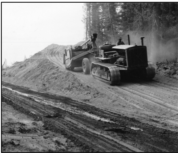
Widening a pumice cut on Rim Road: A 75-HP caterpillar and LaTourneau at work near Station 920 during a 1935-36 construction project. Final Construction Report on Rim Road, PEC-7-C1, Unit 1 Grading & PEC-7-B, 7-C, Widening. WFLHD Archives.
