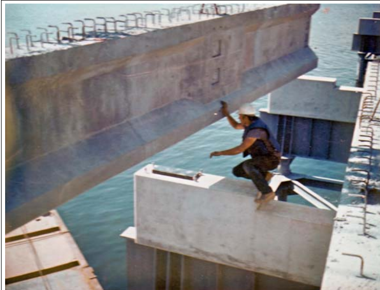
The prestressed beams were set into place “on a 1- or 2-inch rubber pad. The man is one of the contractor employees,” Larry added, “probably an ironworker. I’m not so sure that it isn’t Bill Ayotte’s brother-in-law, Clinton Meyer. ” Photo courtesy Larry Adams.
