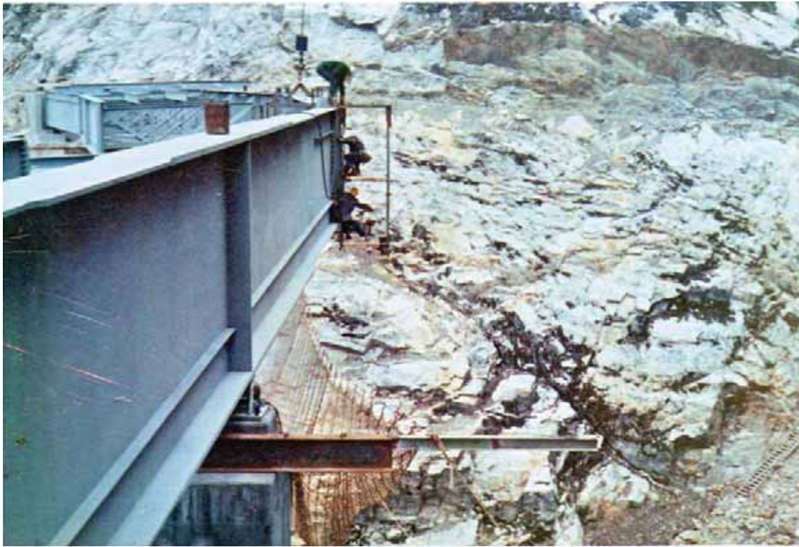
Larry Adams provided these pictures, noting that “This is how we checked the bolts. I’m the one on the bottom with the torque wrench. The others are Ironworkers. I was working with Tom Neunaber on the Horsetail Falls Bridge on the North Cross State Highway.”
