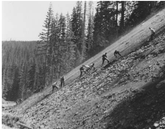
A crew hand-slopes a talus slide on the Santiam Highway (Oregon Forest Highway Project E-23-G1), 1932-34. Photo from Final Construction Report, WFLHD Archives.
