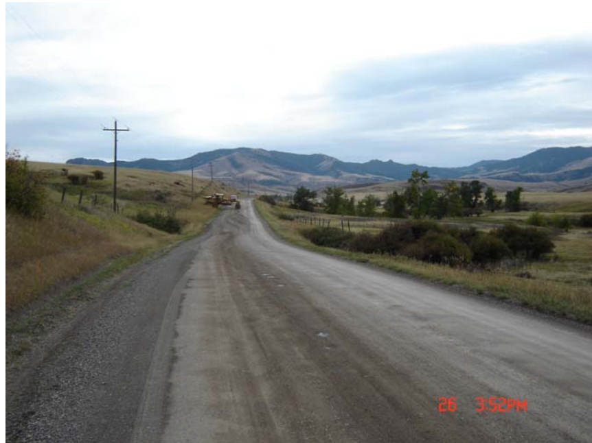
A motor grader works on a missile base road in Montana. WFLHD Construction Photo Archives.
