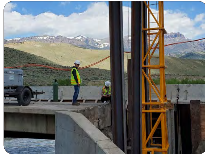
Pictured above, Phillip Clark a participant in the Professional Development Program (PDP) accompanied by CFLHD Project Engineer, Dusty Escamilla perform a Pile Driving Inspection on the Southfork project in Park County, Wyoming. The Southfork Road project was a widening/reconstruction, resurfacing, restoration, rehabilitation (4R) and gravel resurfacing project including a two span concrete bridge. The route is primarily used as recreational access to Shoshone National Forest, and provides agricultural and residential access. — Shoshone National Forest, Wyoming
