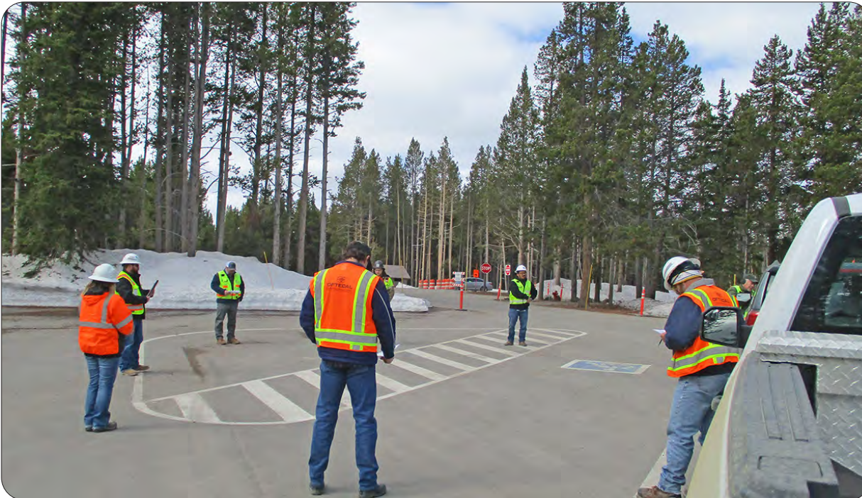
Socially distanced Partner meeting at the Fishing Bridge to Indian Pond East Entrance Road Project site. The project included reconstruction of the road, rehabilitation of Fishing Bridge, drainage work, reconstruction of parking areas and construction of a new parking area within Fishing Bridge Village. — Yellowstone National Park, Wyoming
