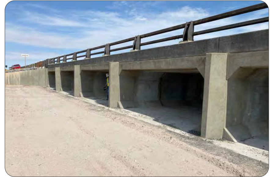
East Fork Concrete box culvert (CBC) completed — Main Park Road, Petrified Forest National Park, Arizona
