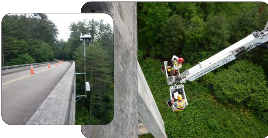
The Bridge Inspection team performs a pier inspection and has been monitoring a wind meter to help the NPS gauge the safety of the aging structure (above left and right). With wind being a critical loading factor on this aging bridge, a wind meter was mounted on the bridge to monitor the wind speeds. A crucial tool in determining when the bridge would need to be closed for safety pending its replacement with a new segmental concrete bridge in Fall 2021. — Laurel Fork Bridge, Blue Ridge Parkway, North Carolina
