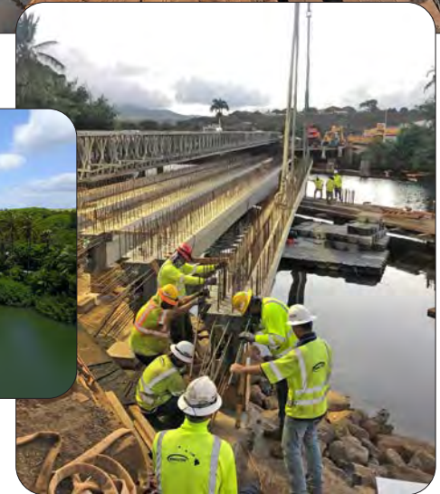
The Hanapepe Bridge project is located on the Kaunualii Highway and crosses the Hanapepe River. The project improves safety and reliability addressing bridge width, load capacity, bridge railing and transitions, bridge approaches and to mitigate the effects of scour. — Kauai, Hawaii
