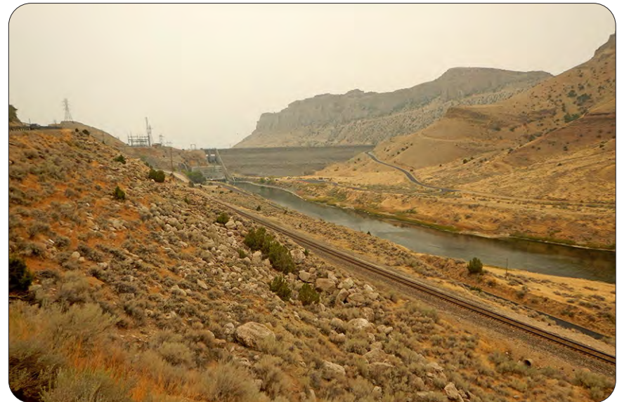
In partnership with the Bureau of Reclamation Wyoming Area Office, CFLHD performed road reconstruction on Boysen Dam Road and the access road which runs between the dam and Upper Wind River Campground. — Boysen Dam, Wyoming
