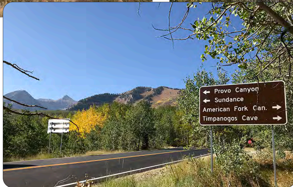
Cascade Springs Road FLAP project consisted of drainage and safety improvements, rehabilitation and paving. — Uinta-Wasatch-Cache National Forest, Utah
