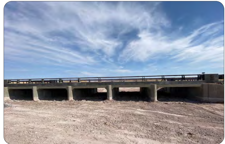
Dry wash concrete box culvert (CBC) completed — Main Park Road, Petrified Forest National Park, Arizona
