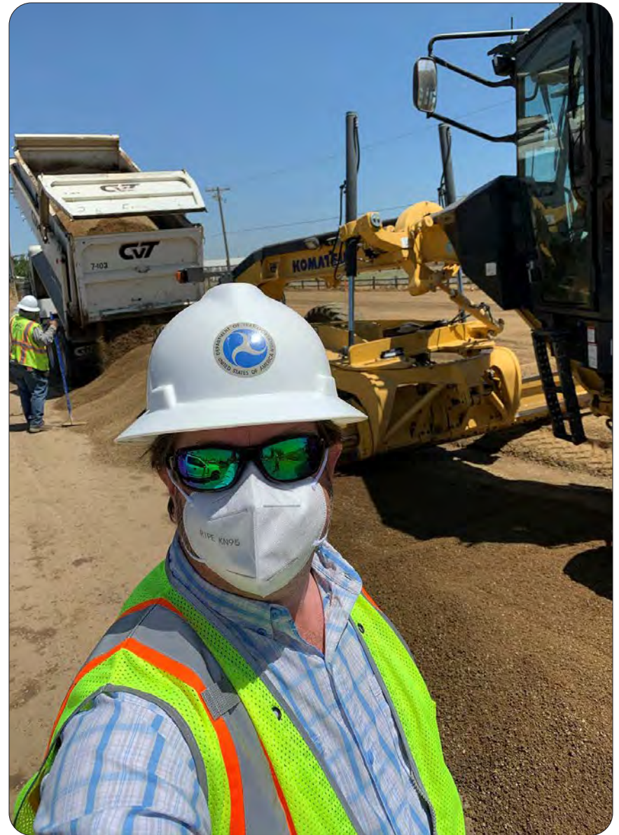
CFLHD Project Engineer, Jack E. Carlson onsite at the Cottonwood Trail Project under the Architectural Barriers Act (ABA) this project provides better access on trails for visitors with disabilities. — Merced National Wildlife Refuge, California
