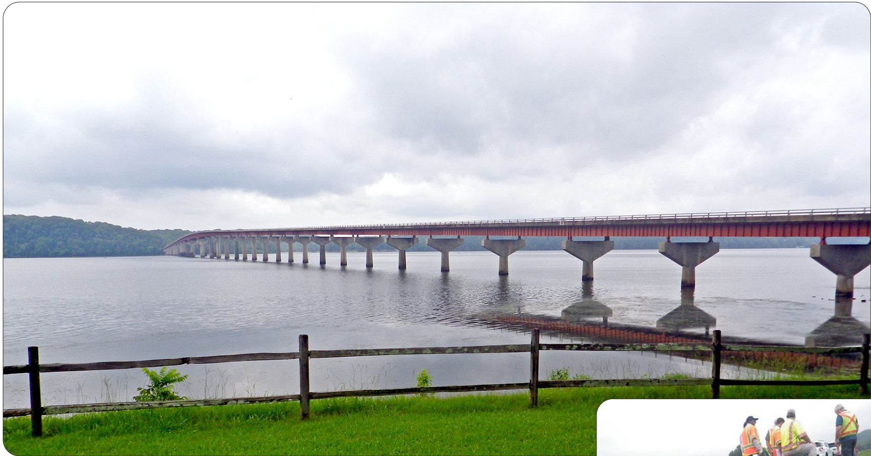
Natchez Trace Parkway Scoping Field Review, John Coffee Memorial Bridge over the Tennessee River — Alabama
