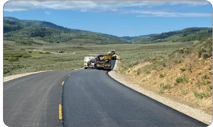
The Strawberry Sheep Creek project consisted of widening, reconstruction, and paving of the unpaved portion (12.3 miles) of Forest Routes 70131, 70042, and 70051, known as the Strawberry Sheep Creek Connector. Work also included drainage and safety improvements. — Uinta-Wasatch-Cache National Forest, Utah
