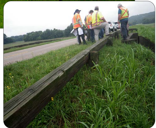
Scoping Field Review, Timber Guardrail at Natchez Trace Parkway Underpass Animal Crossing — Tennessee
