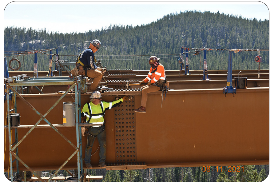
Beartooth Highway reconstruction project addressed approximately 2.32 miles of US 212, and improved roadway alignment and grade. The project also included removal and replacement of an existing bridge, and construction of a new 36 foot wide bridge. In addition, this project covered improvements to the West Summit Site on the highway east of the roadway improvement project at Beartooth Pass, to include grading and installation of aggregate base to the entrance road and parking area. — Shoshone National Forest, Wyoming
