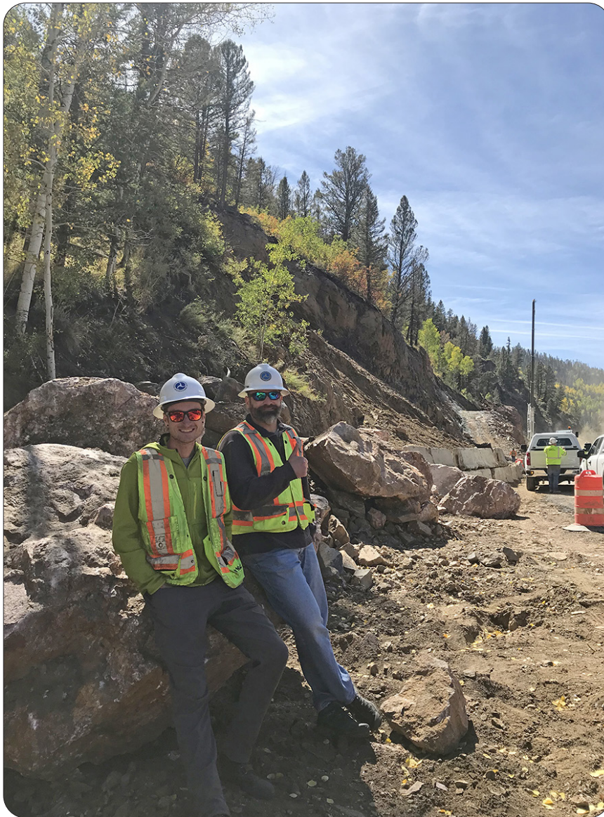
Left: Brendan McGarity, & Dominic Monarco, both Geotechnical Engineers onsite at the US50 Little Blue Creek Canyon Project — Colorado DOT, FHWA and CFLHD, in cooperation with the FS, Grand Mesa Uncompahgre and Gunnison National Forests, BLM, and NPS, are improving 3.8 miles of U.S. Highway 50. The route provides access to various federal lands, including The Black Canyon of the Gunnison National Park, Curecanti National Recreational Area, BLM and FS land. — Colorado
