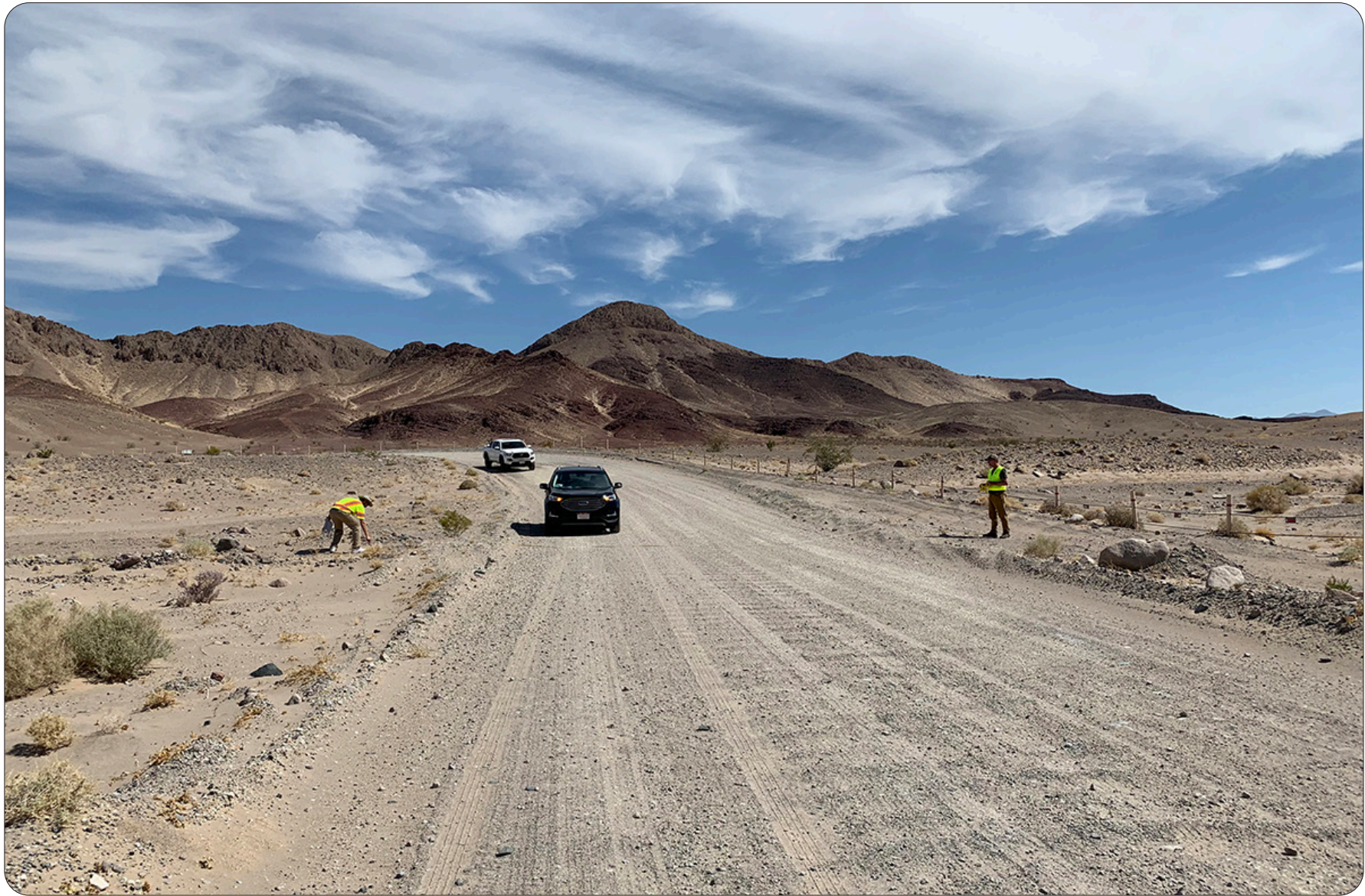
Dumont Dunes Road rehabilitation project during 70% Field Review. In this location of the project we are shifting the proposed roadway improvements slightly toward the inside of the horizontal curve and adding curve widening. Michael Daigler, Project Manager (left) assisted by the contractor Project Manager (right) are measuring across the roadway to determine the best fit for the proposed improvements while taking into account how to minimize impacts to the environment. Slightly out of the shot to the right there is an OHV (Off-highway Vehicle) trail that must not be impacted by the project. — Dumont Dunes Road, Mojave Desert, California
