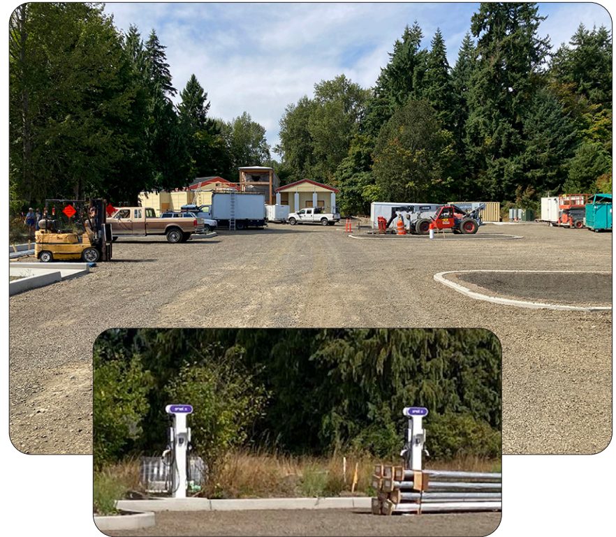
Dungeness River Audubon Center parking lot under construction and equipped with electric vehicle charging stations. TTP funds were utilized by the Jamestown S’Klallam Tribe to construct the parking lot and driveway access. — Clallam County, Washington
