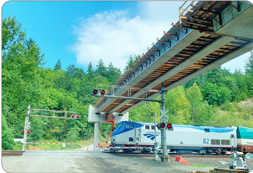
Ridgefield National Wildlife Refuge bridge replacement project removed an existing single lane timber trestle bridge and an at grade railroad crossing, replacing it with a new concrete bridge over Lake River and the railroad, providing safe and reliable crossing via rail and river — River S Bridge over Lake River, Ridgefield, Washington.
