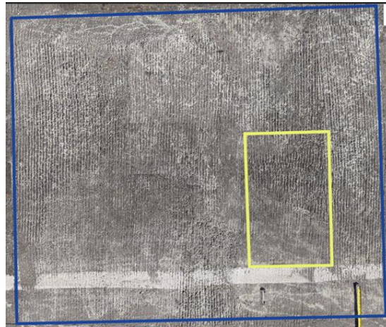
Figure 4.6 Delamination in a Repair Patch Marked with Yellow Box (P6)
