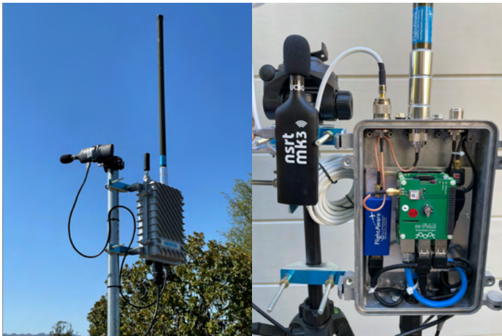
Figure 4. Sensor controller rooftop deployment with ADS-B and a SLM (left). Sensor controller components (right).
