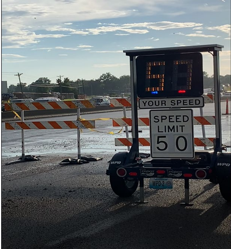
Figure 3-8. Speed trailer with red and blue lights in field study
