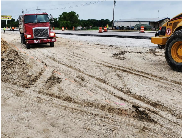
Figure 20. DAL-SH 121 Detour, Soft Subgrade Rutting under Construction Traffic.
