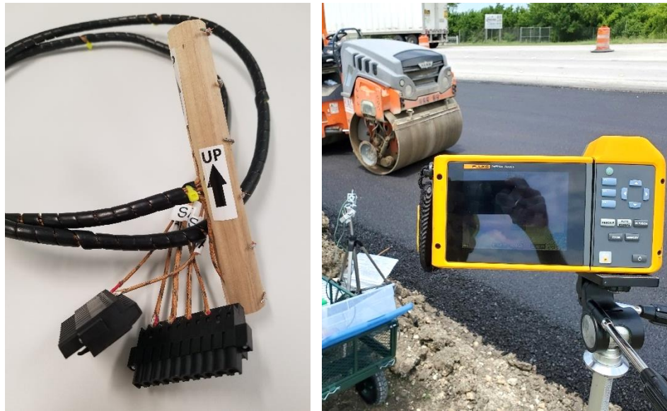
Figure 23. Temperature Probe, Installation Site, and IR Camera.
