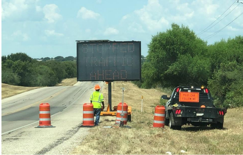
Figure 16. PCMS Displaying STOPPED TRAFFIC AHEAD Message.
