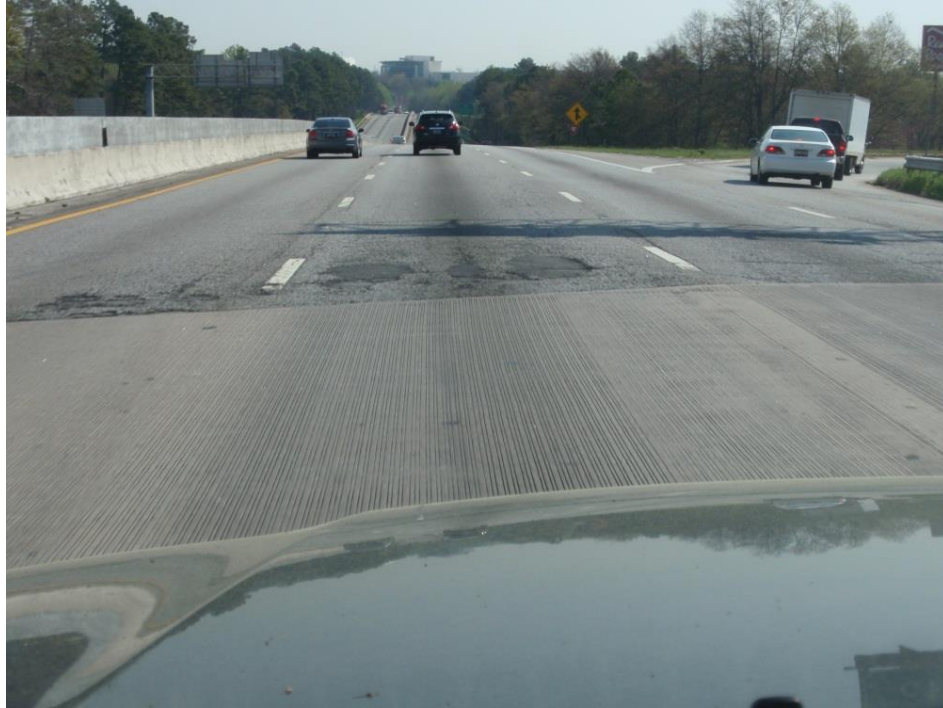
Figure 2.3. Raveling of OGFC on I-85 in Greenville, SC
