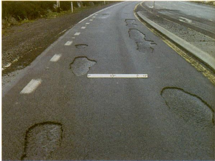
Figure 2.2. Delamination Distress in an Asphalt Pavement (National Association of Australian State Road Authorities, 1987).
