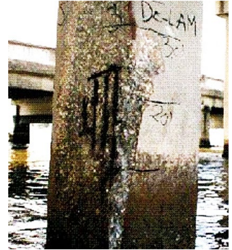
As corrosion of steel reinforcing bars proceeds, it can cause cracking and loss of concrete.
