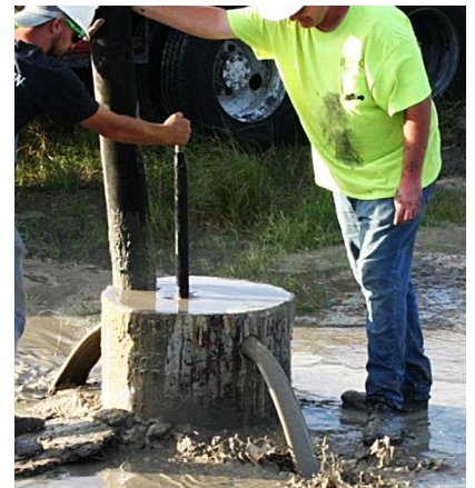
Slurry pours out of a steel collar as cement is piped into a drilled shaft excavation.
