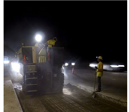
Slab replacement crews often work at night to reduce the time that lanes are closed to traffic.
