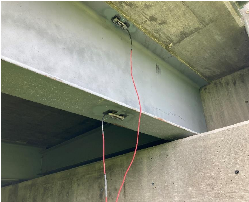
Figure 52. Strain gauges at abutments
