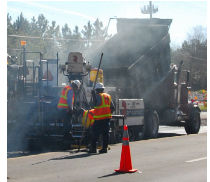
Hot-mix asphalt is continuously placed into the path of a paving machine as part of a road resurfacing operation.
