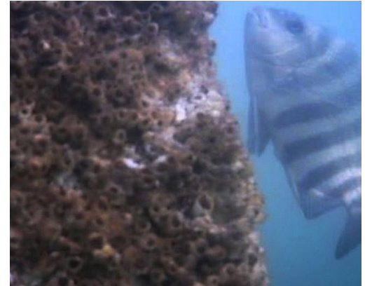
Underwater structures are often colonized by barnacles and other marine life, which can host bacteria that are destructive to steel.
