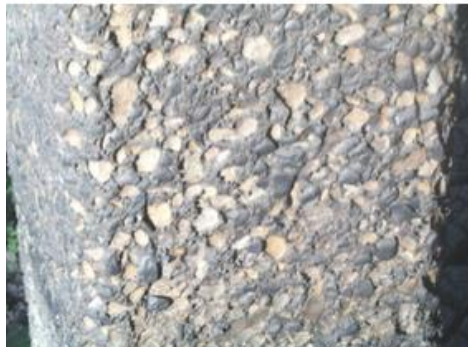
Figure 2.2. Microbial-induced Bio-deterioration of Concrete. (Trejo et al., 2008).
