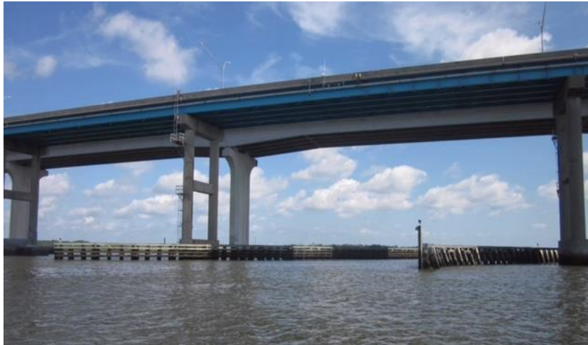
Figure 1.1. Picture of a Florida bridge over Matanzas River with Corrosion of Steel Piles.
