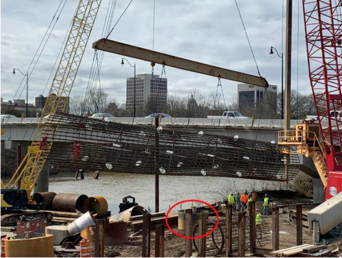
Figure 3. Photo. Location of drilled shaft near the bank of the Ocmulgee River
