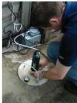
Routing recess for the expandable ring in preparation for CAPO-TEST to evaluate surface strength of an industrial floor slab
