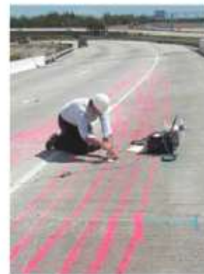
Testing for quality of grout injection in cable ducts located by ground penetrating radar
