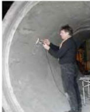
Detection of delaminations and honeycomb in sewer pipe
