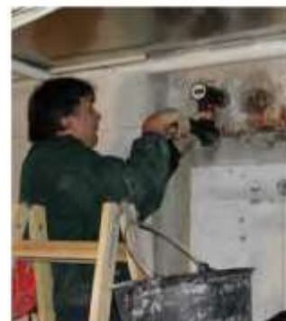
CAPO-TEST being performed in parking garage to evaluate in-place strength of suspect concrete
