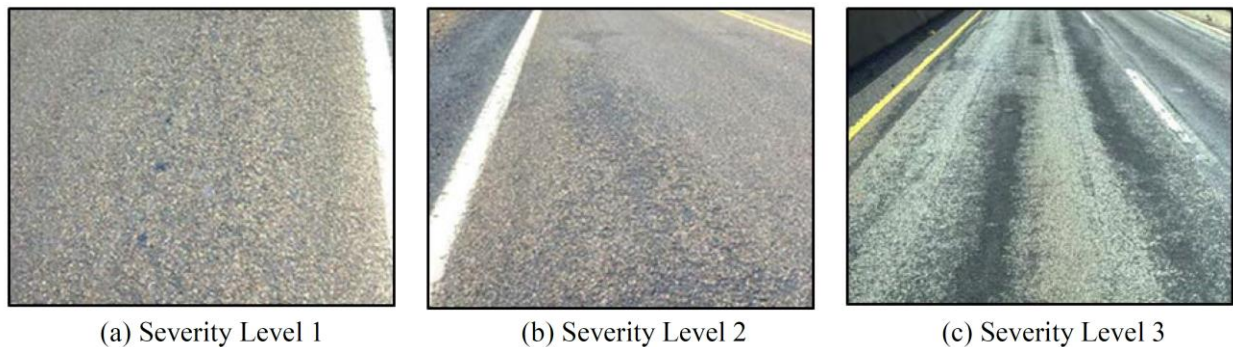
Figure 4. Raveling classification in GDOT (GDOT, 2017).
