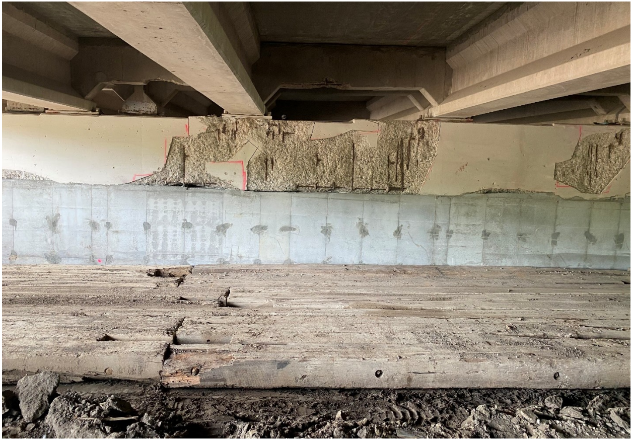
Figure A.6. Spalling and delamination on north side of the west face of Pier 12WB
