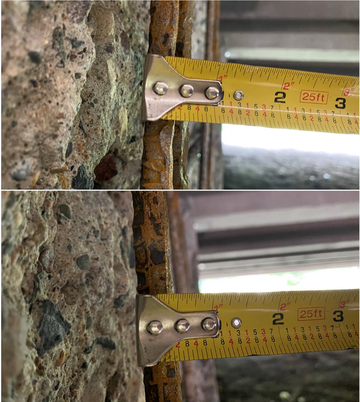
Figure A.18. Exposed stirrups on south end of the west face of Pier 15EB, with rebar diameters of 3/8" and 7/16", respectively
