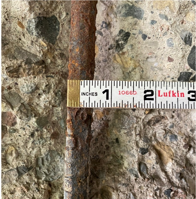
Figure A.8. Corroded stirrup rebar diameter 9/16" on west face of Pier 12WB
