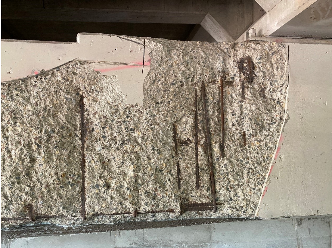
Figure A.7. Spalling on west face of Pier 12WB showing longitudinal and stirrup rebar
