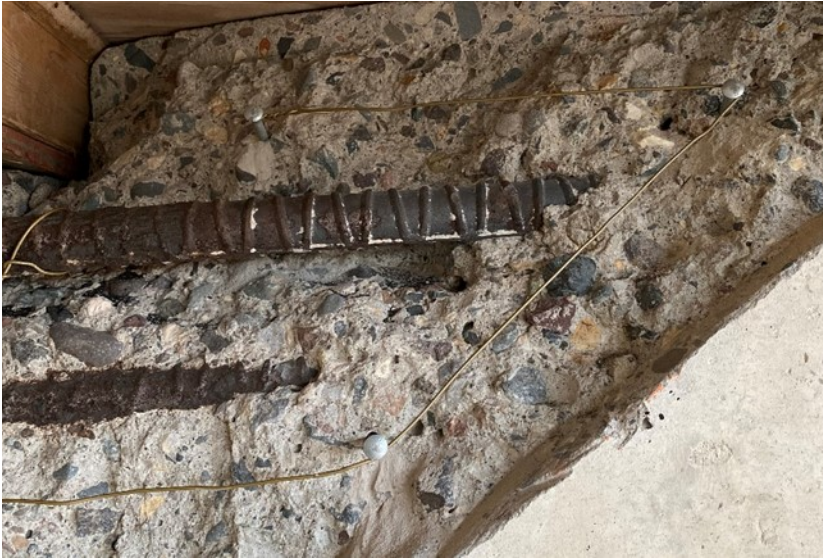
Figure A.44. Exposed longitudinal bars with little corrosion on the east face of Pier 48EB
