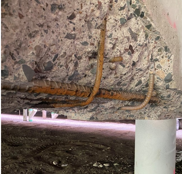
Figure A.12. Exposed rebar to the north of pile 3 on Pier 15EB
