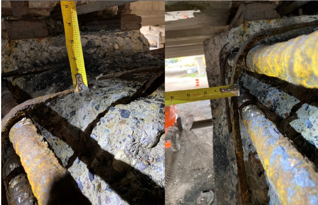
Figure A.39. Severely corroded stirrups, broken over top of Pier 48EB, and diameter reduced to approximately 1/2" on the east side
