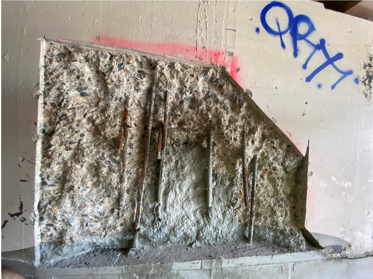
Figure A.3. Spalling on south end of east face Pier 12WB
