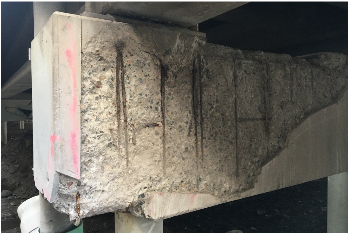
Figure A.17. North end of west face of Pier 15EB showing corner and face spalling as well as delamination on the top of the pier
