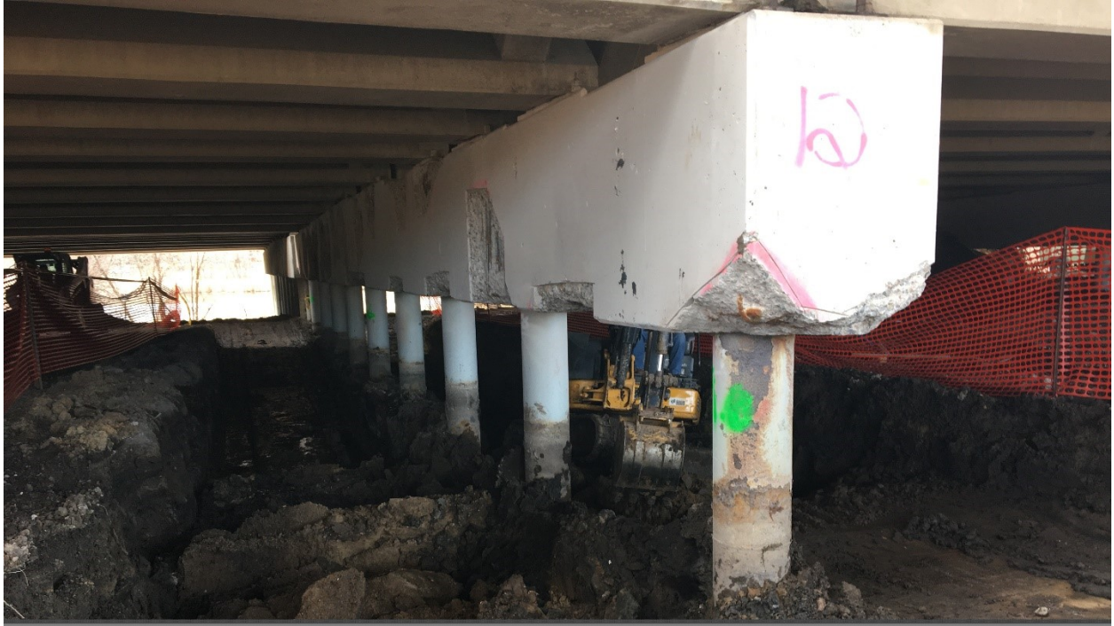
Figure A.9. North end of Pier 12WB showing significant spalling on corners and exposure of longitudinal and stirrup rebar
