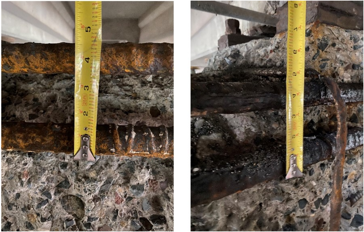
Figure A.42. Corroded longitudinal bars in area shown in Figure A.37, with rebar diameters of about 1 1/2"
