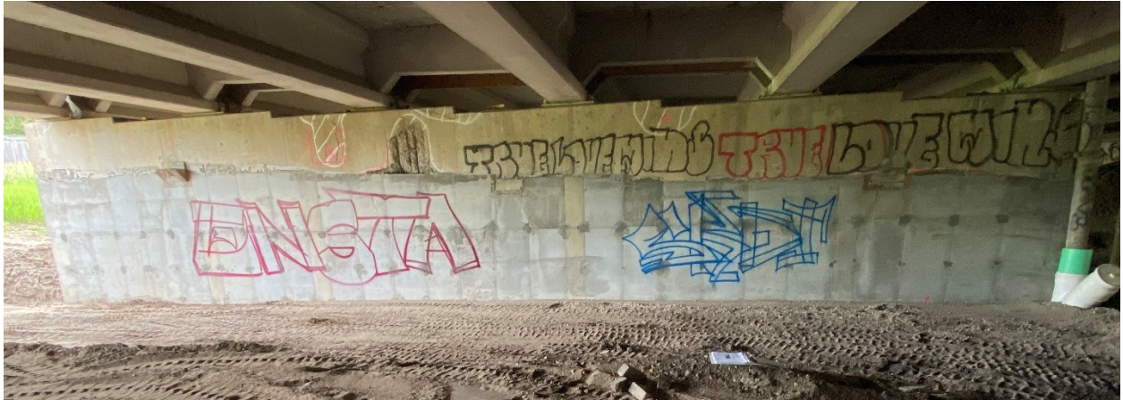
Figure A.25. East face of Pier 21EB showing pier encapsulated in RC
