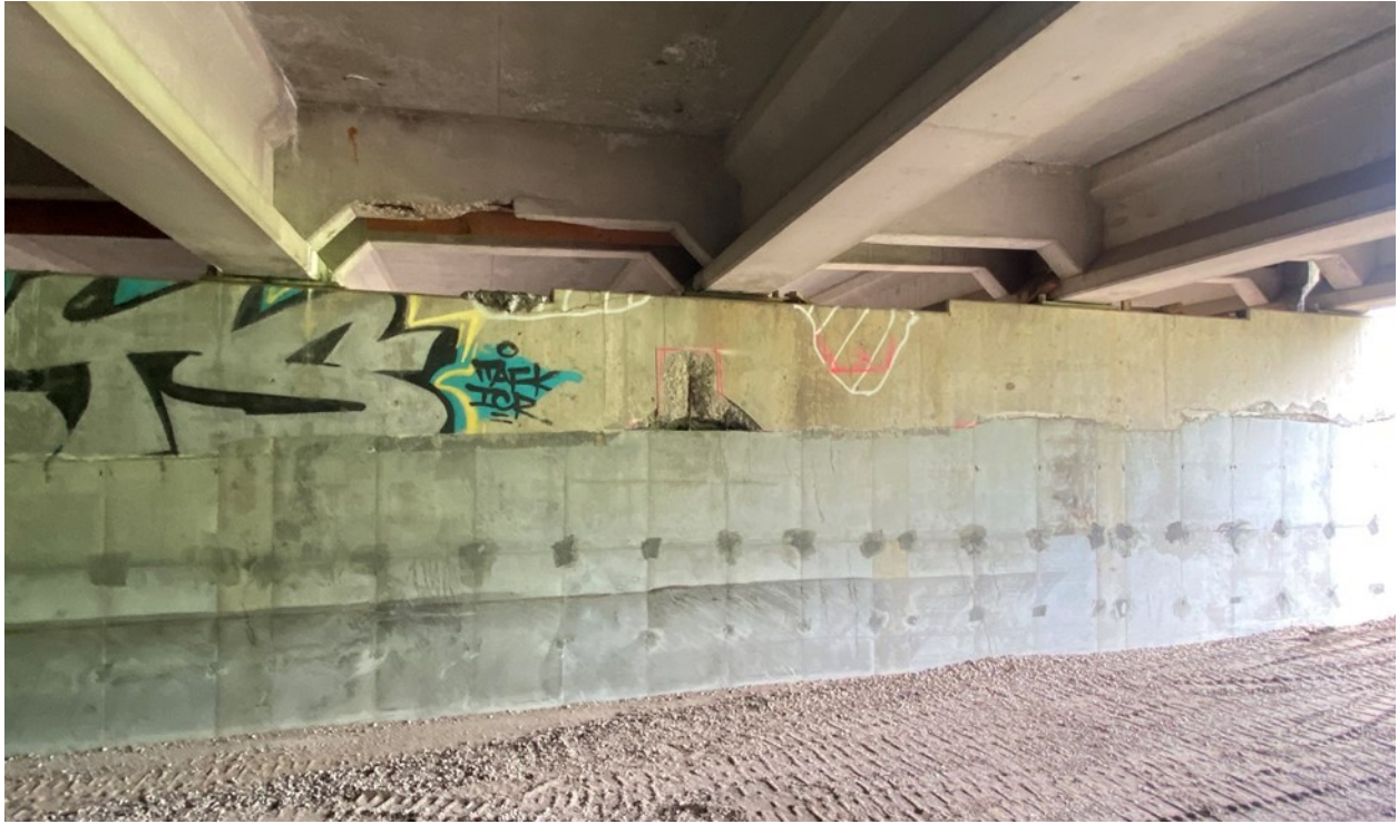
Figure A.30. North end of west face of Pier 21EB showing one area of spalling with exposed rebar
