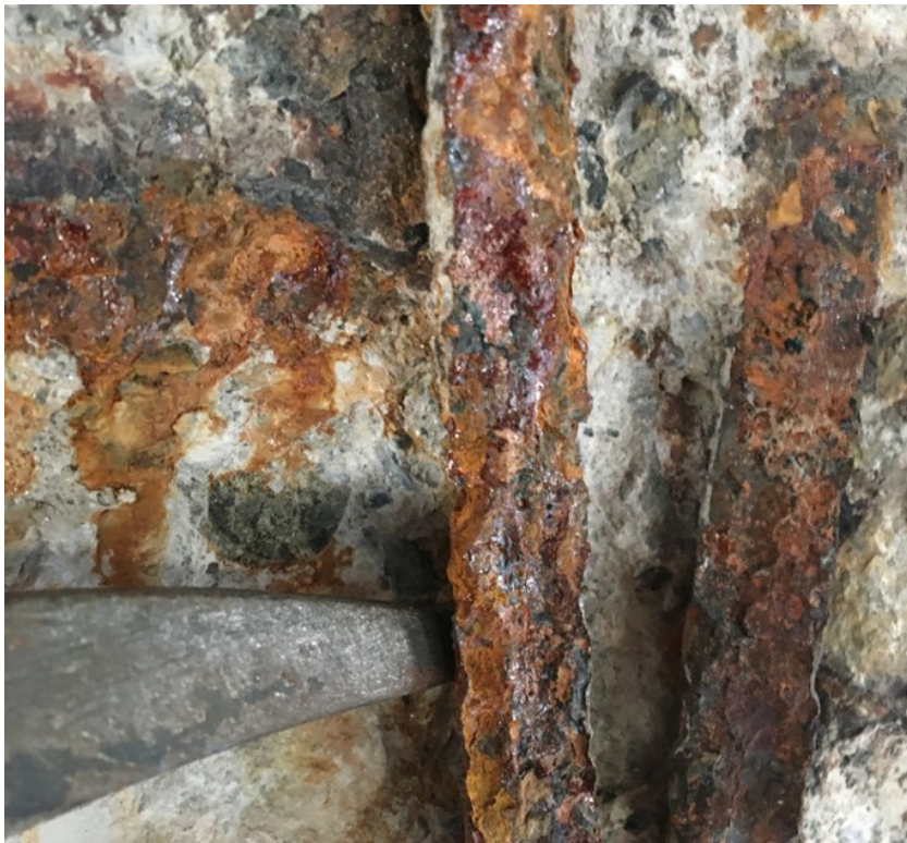
Figure A.24. Severely corroded rebar specimens from south end of Pier 15EB
