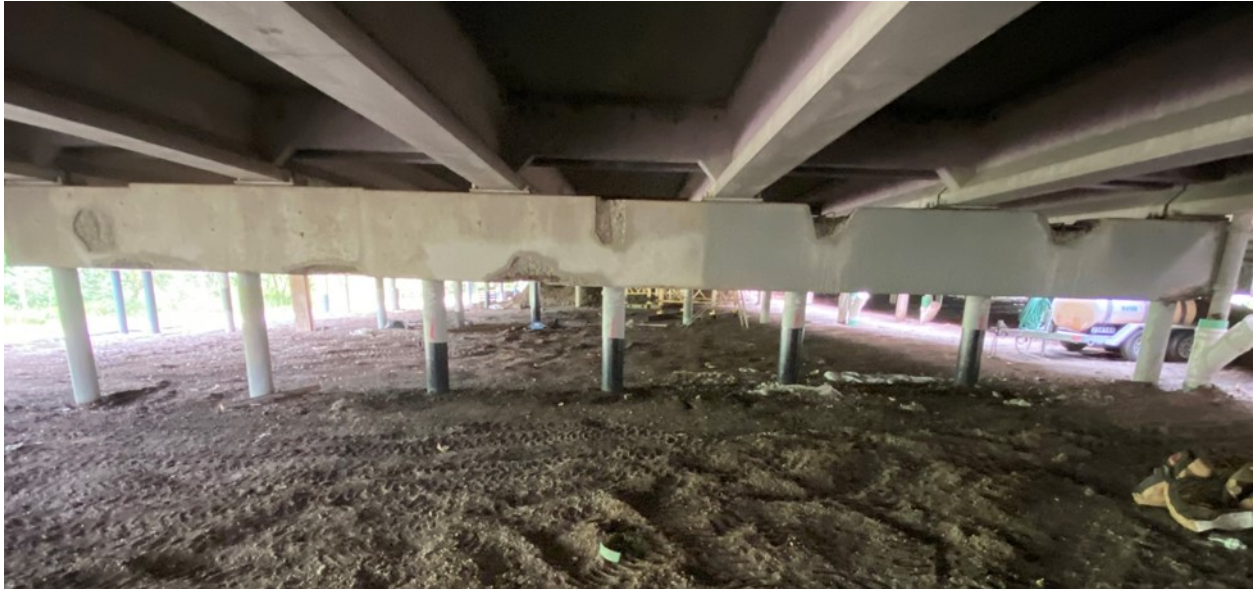
Figure A.10. East face of Pier 15EB showing significant areas of delamination on top of the pier between beams on south side of beam and on bottom of the pier on the north side of the beam
