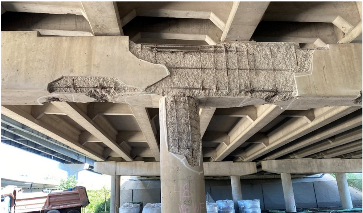
Figure A.34. Close-up of delaminated area in the center of the west face of Pier 48EB
