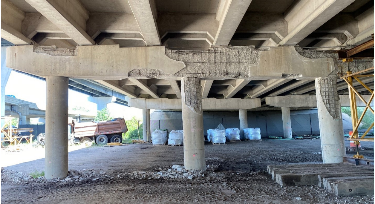
Figure A.33. West face of Pier 48EB showing delamination between multiple columns and on the columns themselves
