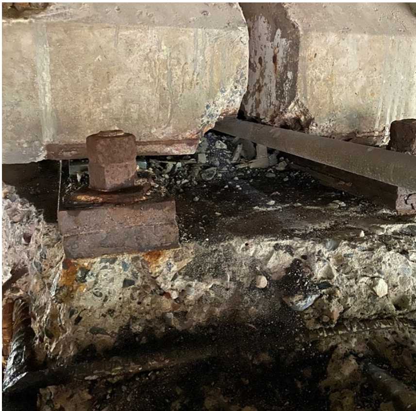
Figure A.40. Connection on top of Pier 48EB showing corrosion on the connecting plates and bolts
