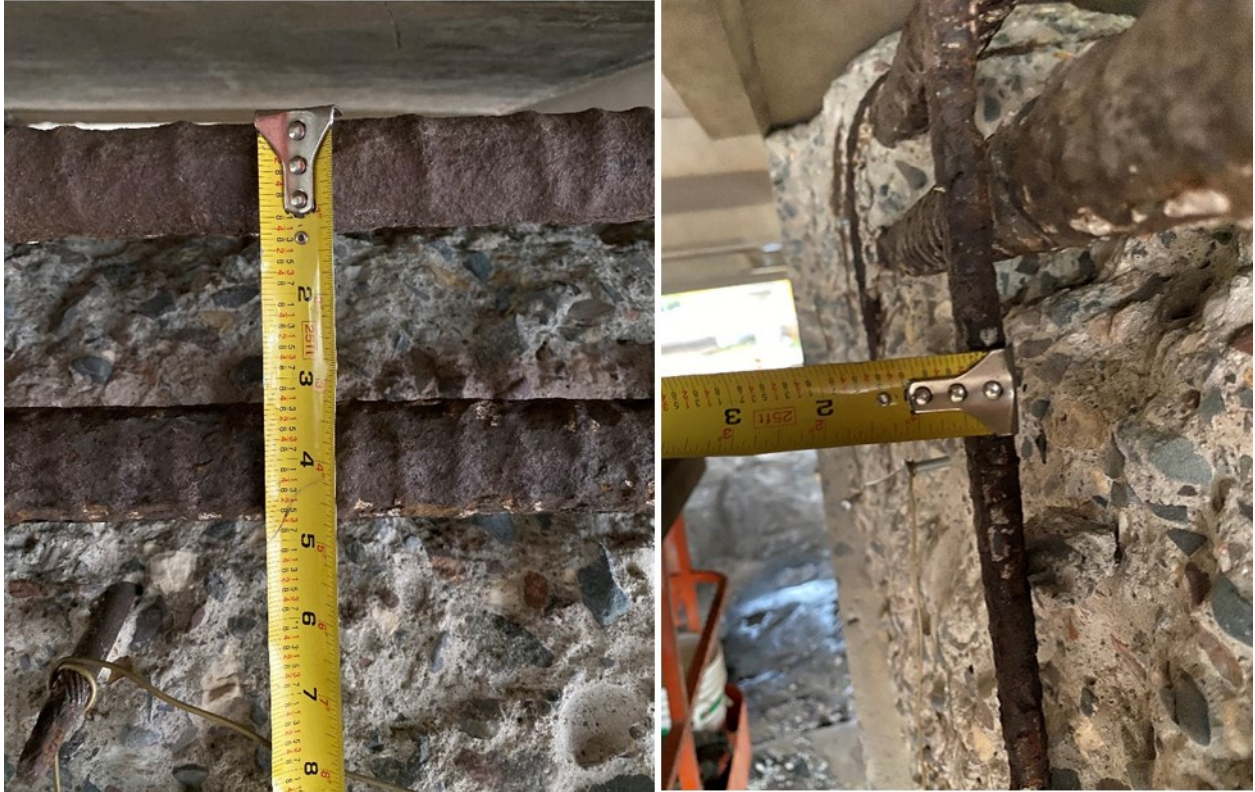
Figure A.45. Exposed rebar with mild corrosion from area in Figure A.37, with rebar diameters of 1 1/2" and 1/2", respectively
