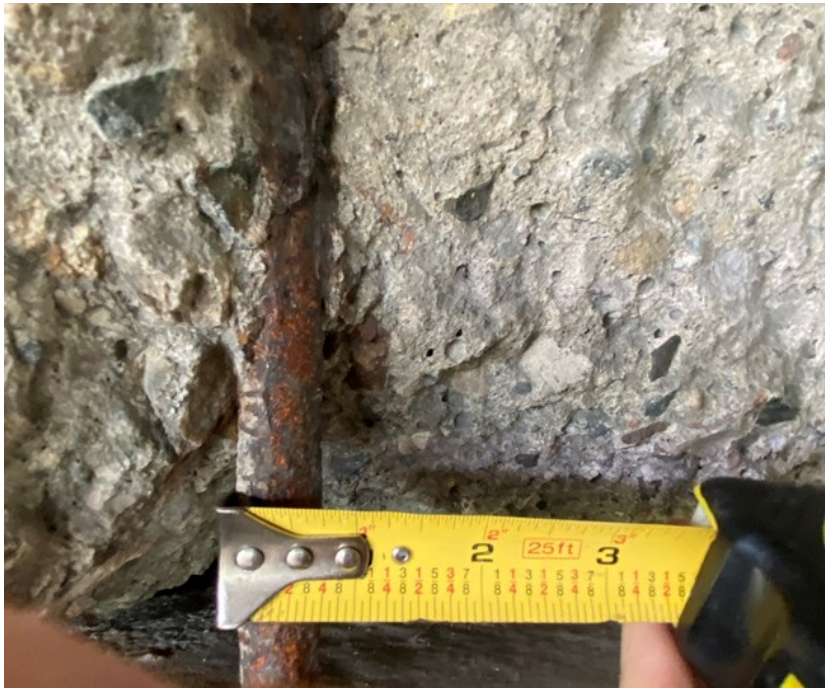
Figure 28. Exposed corroded rebar with diameter of 3/4"
