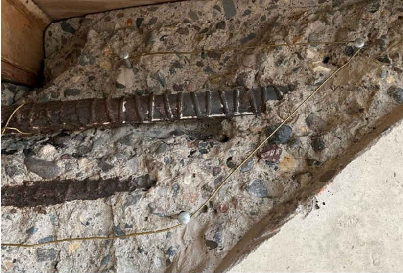
Figure A.43. Delaminated area shown in Figure A.37 from the east side of Pier 48EB
