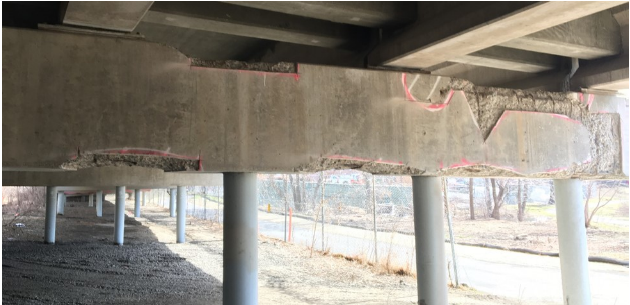
Figure A.22. West face of Pier 15EB showing multiple spalling and delamination areas at north side of the pier
