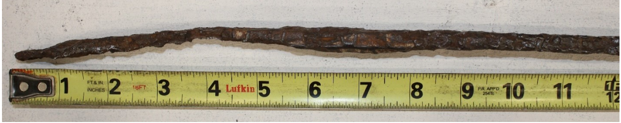
(f) S6 sample, #5 bar (15% total section loss, 90% pitted end)
