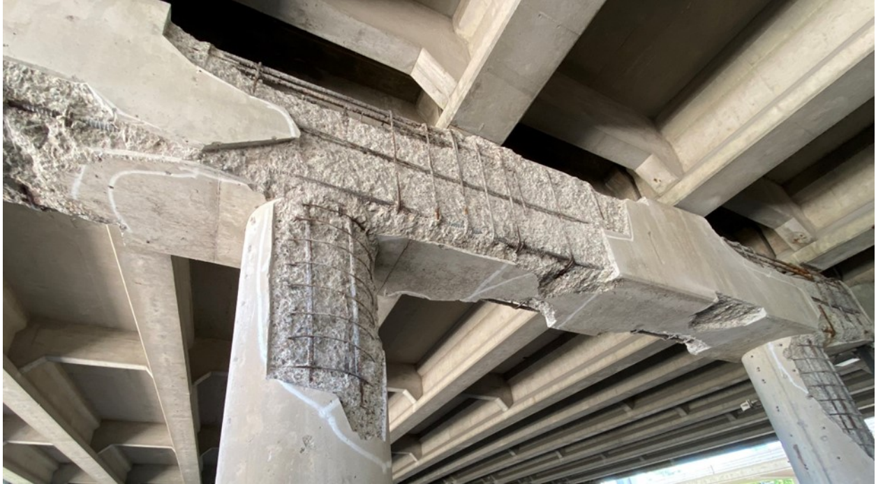
Figure A.35. Underneath angle showing severe delamination on Pier 48EB
