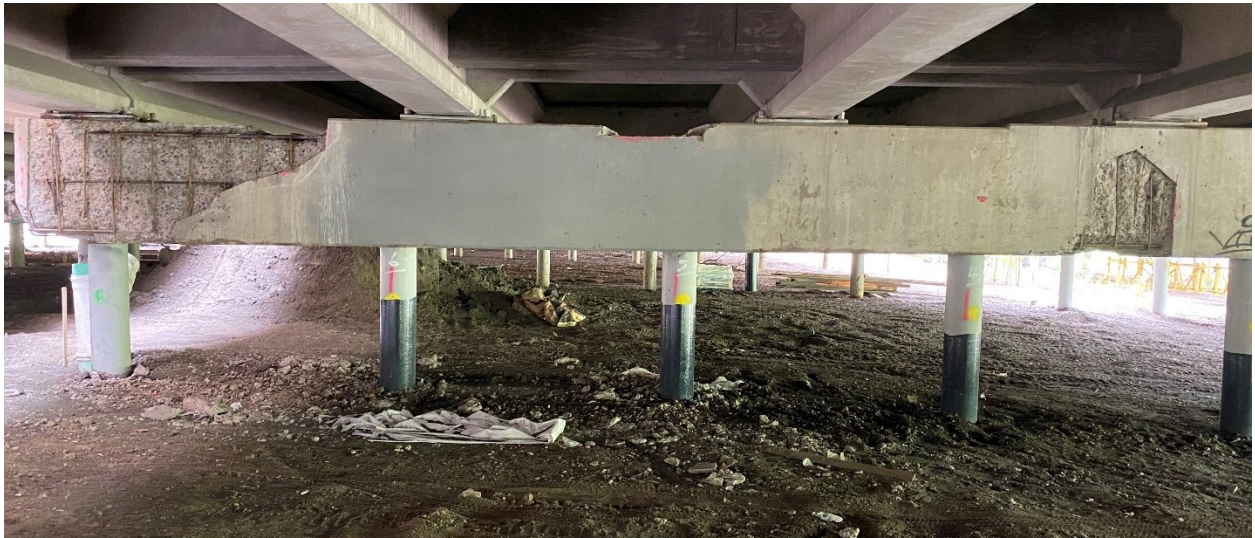
Figure A.15. West end of Pier 15EB showing two areas of spalling, with entire south corner having rebar exposed nearly to pile 6
