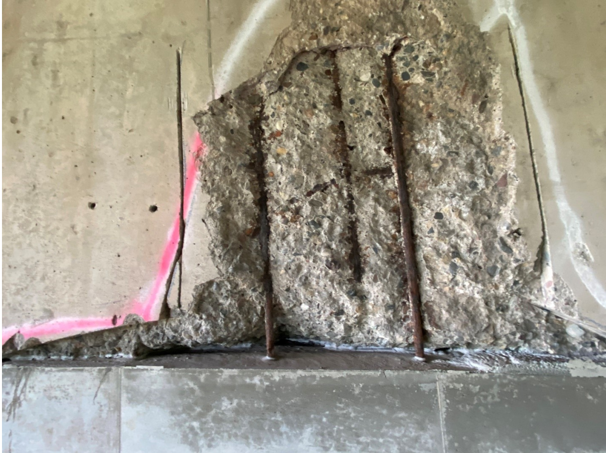
Figure A.27. Area of spalling on east face of Pier 21EB where stirrup rebar is exposed
