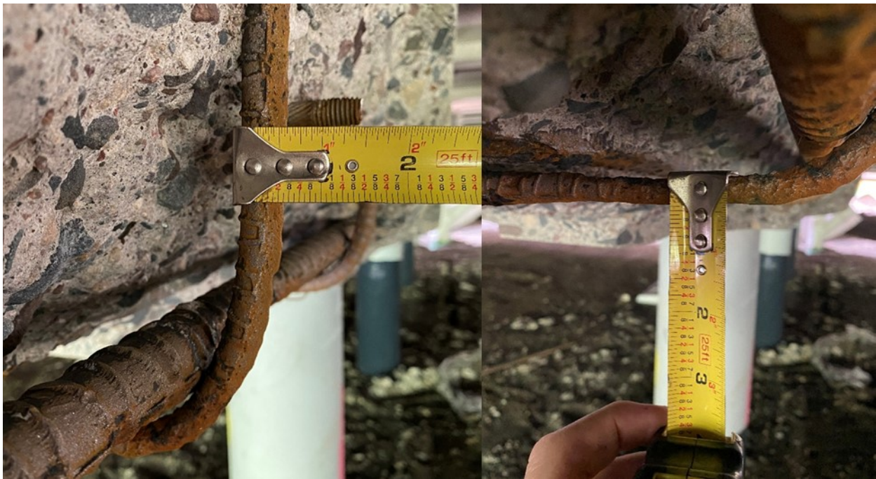
Figure A.13. West face of Pier 15EB showing notable spalling on south end of the pier, delamination on top of beam above pile 5
