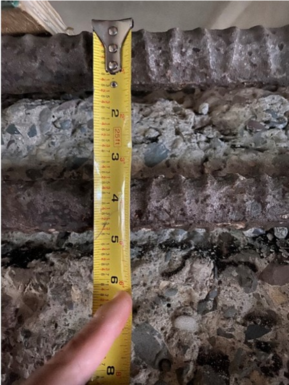
Figure A.38. Exposed longitudinal and stirrup rebar with minimal corrosion from section shown in Figure A. 37, with rebar diameters of about 1/2" and 1 1/2", respectively
