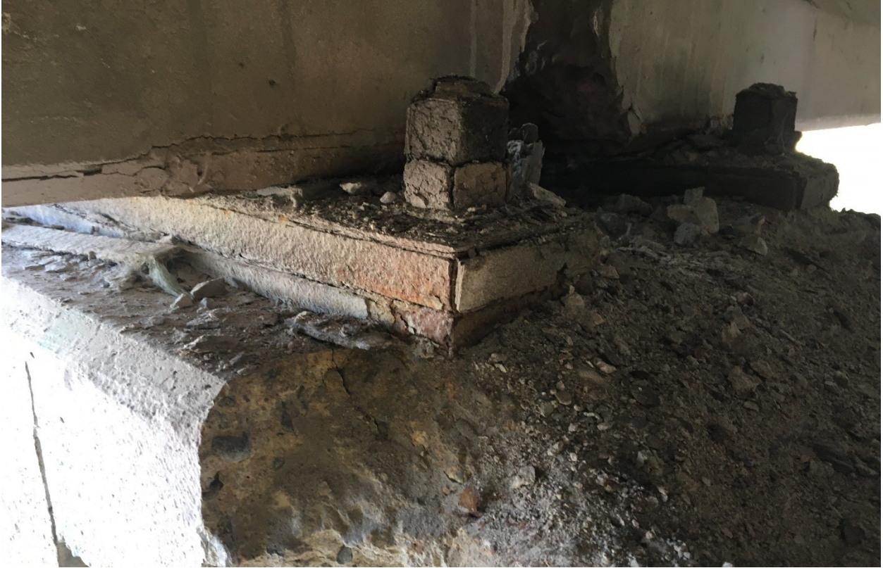
Figure A.19. Top of Pier 15EB at north-most beam connection, with connections showing extreme deterioration and corrosion and spalling evident at top of pier
