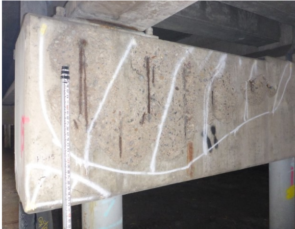
Figure 4.18. Very thin bars between Beams 7 and 8 in Pier 15EB
