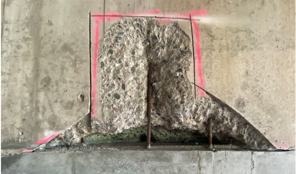
Figure A.31. Spalling with exposed stirrups on west face of Pier 21EB
