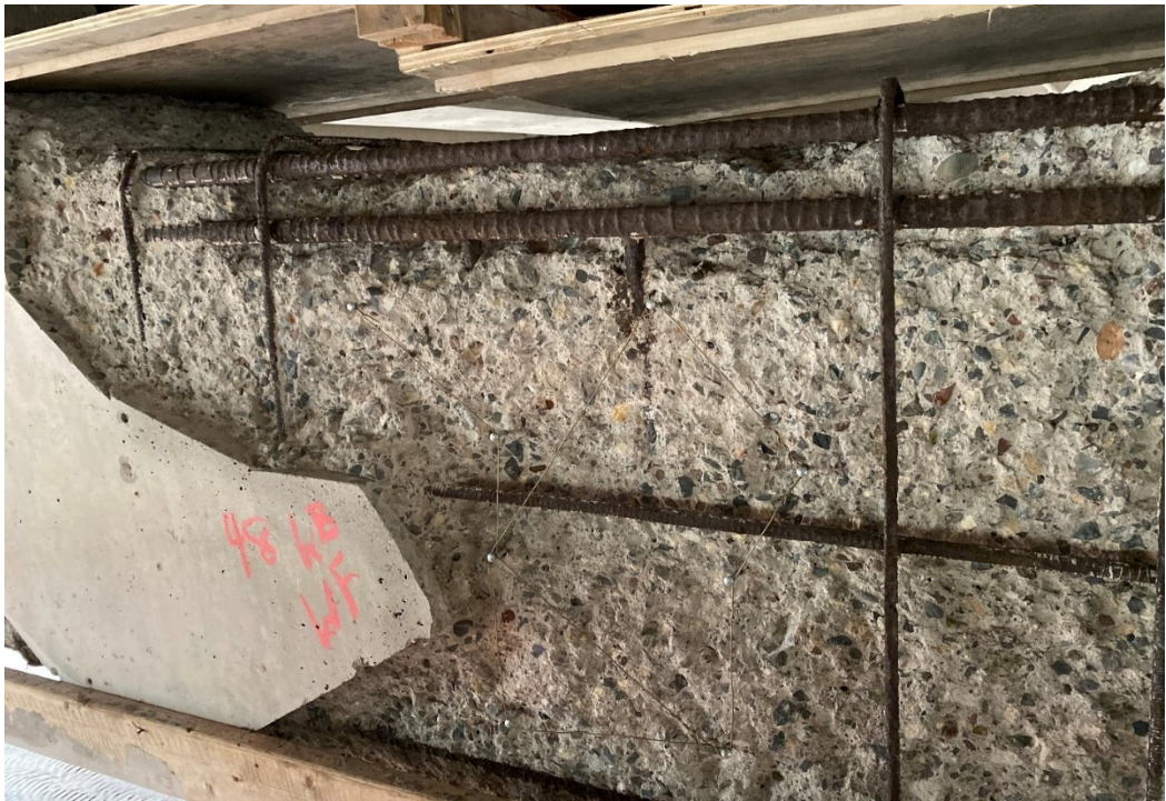
Figure A.46. Additional delaminated area on the west face of Pier 48EB
