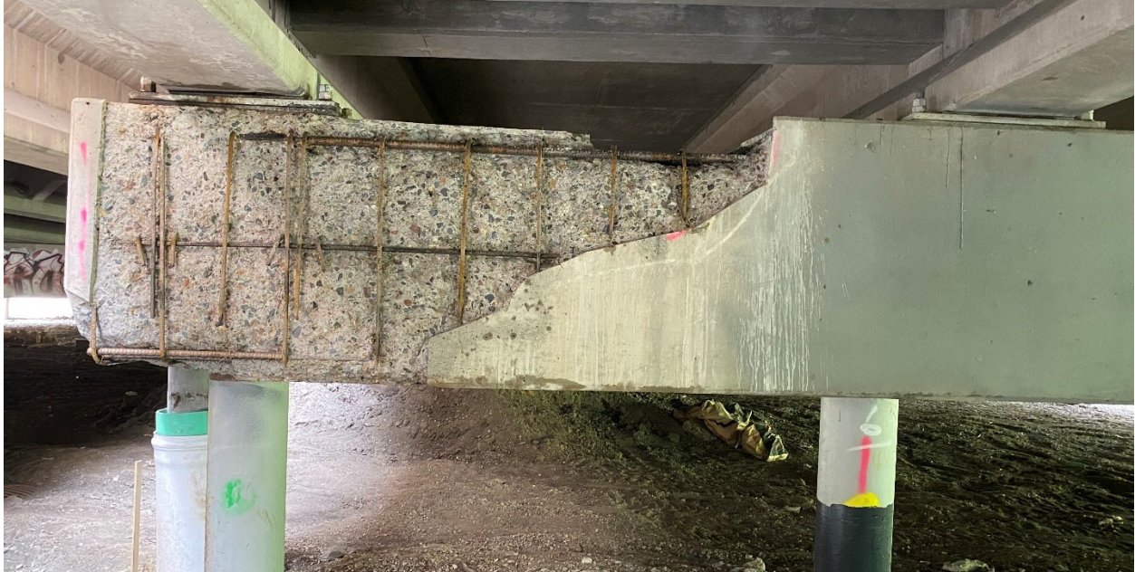
Figure A.16. South end of Pier 15EB showing nine stirrups and all longitudinal rebar on the west face entirely or partially exposed, as well as delamination on top and bottom of pier, most notably on the top near the midpoint of the two piles
