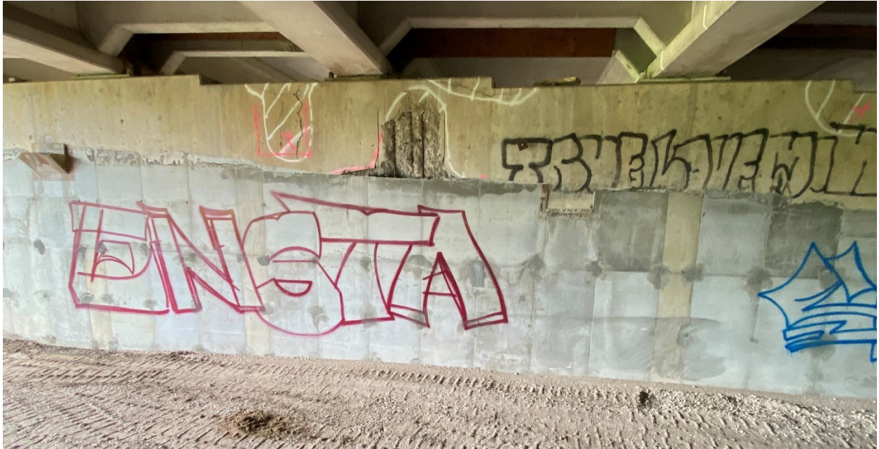
Figure A.26. Northern side of the east face of Pier 21EB showing spalling where concrete has fallen off as well as areas where concrete was retained during spalling
