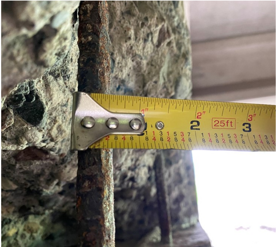
Figure A.32. Exposed corroded rebar with diameter of 1/2"
