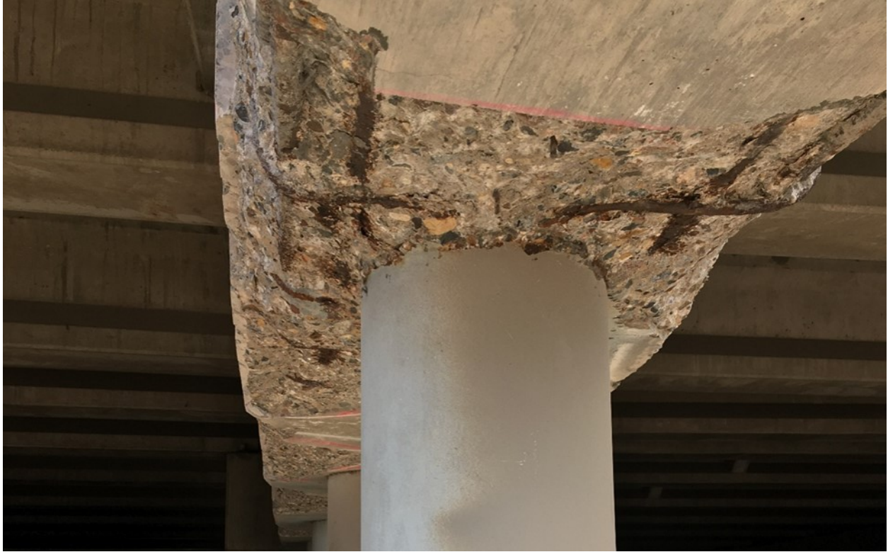
Figure A.21. Underneath Pier 15EB at pile 1, with rust stains present and spalling exposing longitudinal and stirrup rebar
