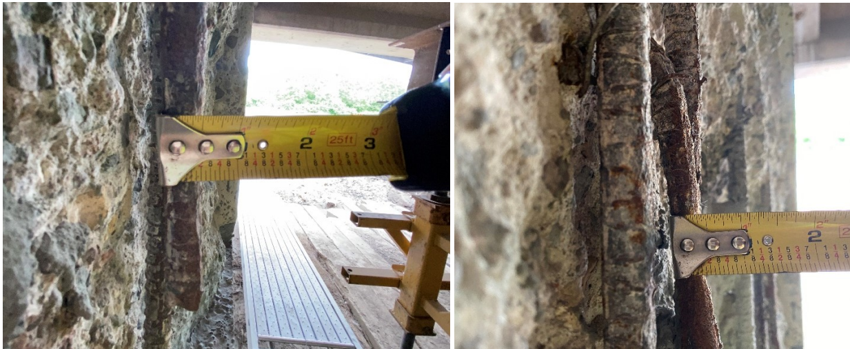
Figure A.4. Rebar section loss in spalling, east face Pier 12WB, with rebar diameters approximately 1/2" and 3/8", respectively
