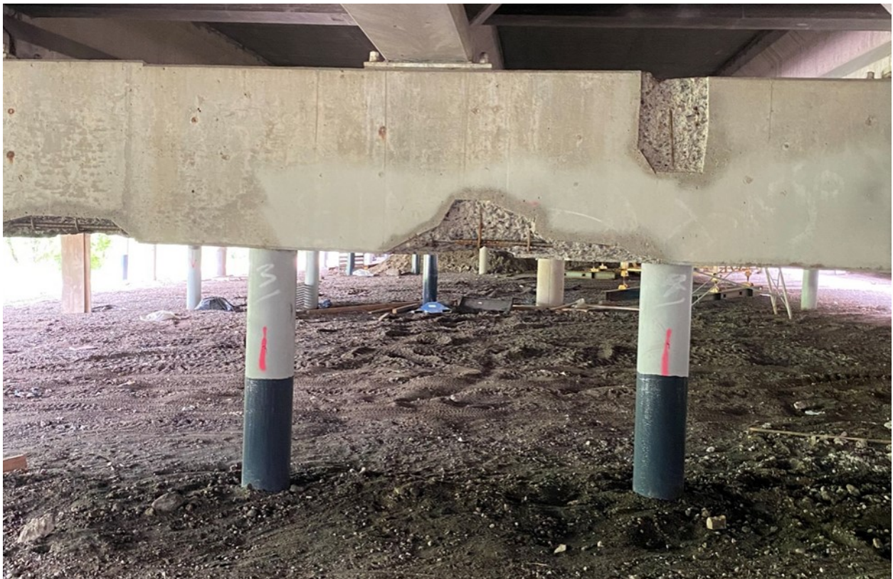
Figure A.11. Spalling and delamination on east face of Pier 15EB showing exposed longitudinal and stirrup rebars between piles 3 and 4
