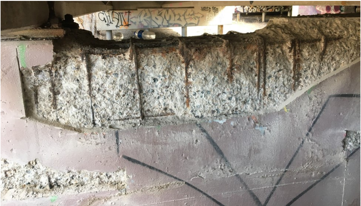
Figure A.20. Spalling and delamination at north end of Pier 15EB
