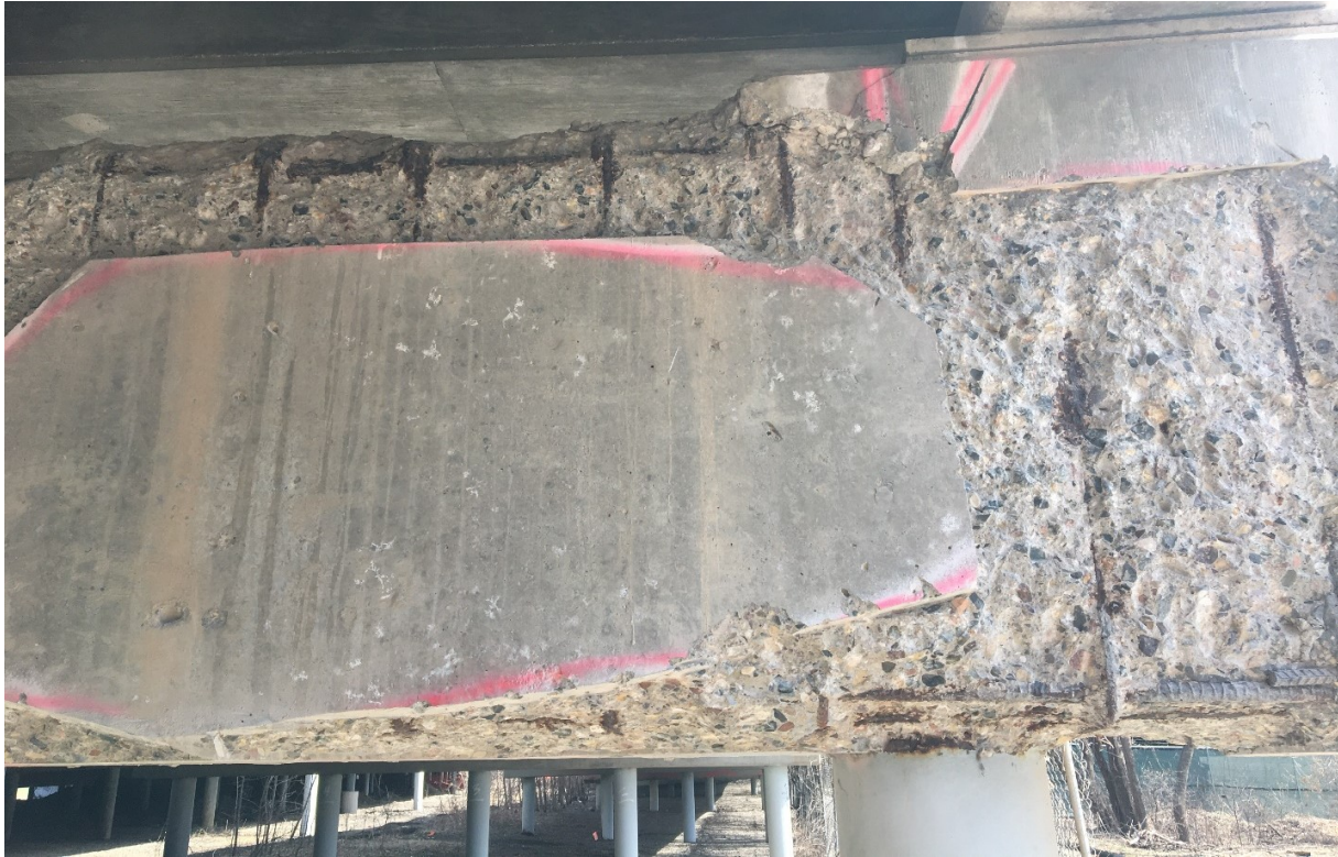
Figure A.23. South end of west face of Pier 15EB showing spalling on face of the pier, delamination on top and bottom of pier
