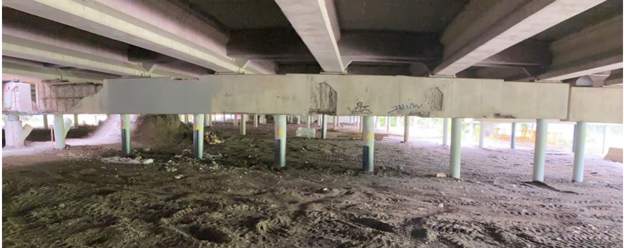
Figure A.14. Vertical and horizontal portions of exposed stirrup shown in Pier 15EB Figure A.3, with rebar diameters of 19/32" and 3/8", respectively
