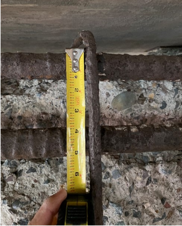
Figure A.47. Exposed rebar in area from Figure A.46, showing both stirrups and longitudinal bars
