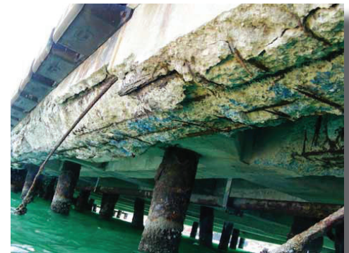
Corrosion of reinforcing steel in concrete structure
