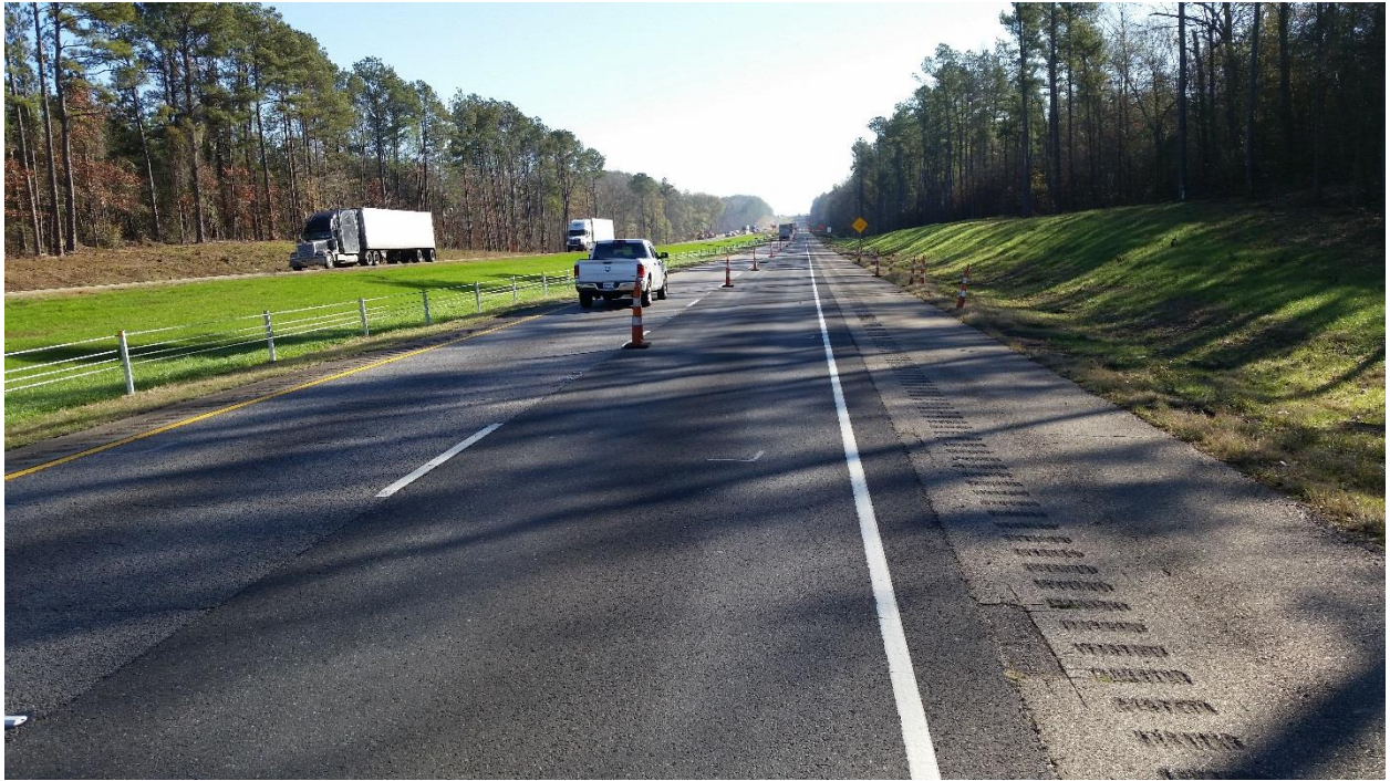
Figure 2 I-20 eastbound lane rutting
