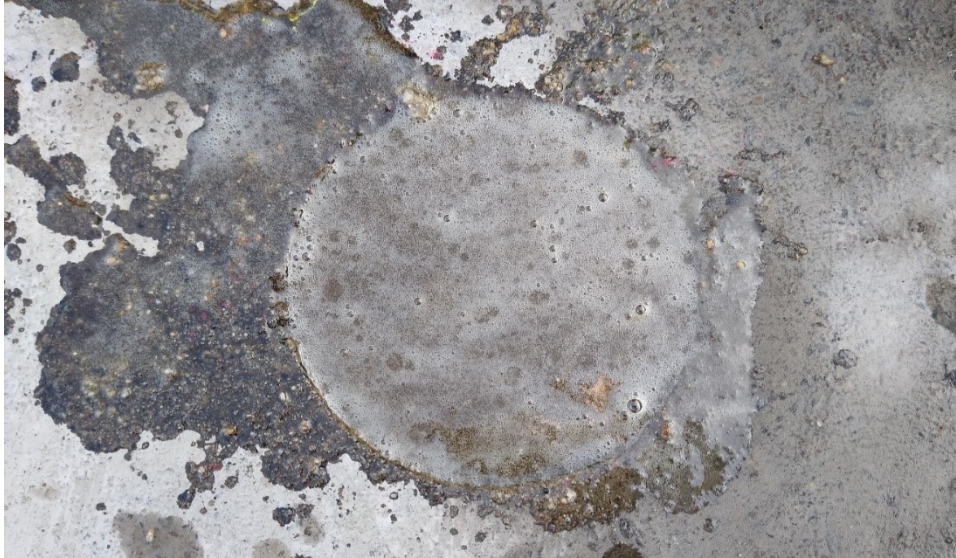
Figure B.7: Filled core hole.
