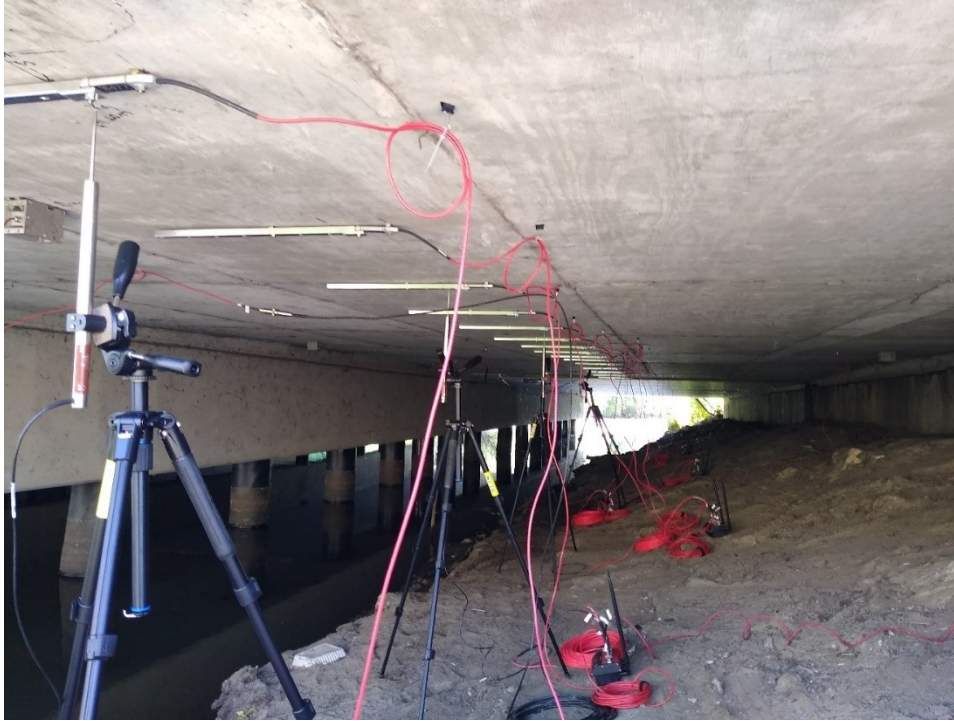
Figure F.5: Array of LVDTs, strain gauges, nodes, and tiltmeters installed on the West span of Bridge 27926.
