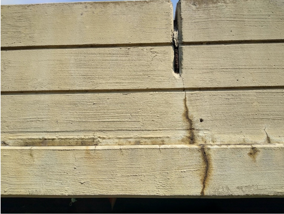
Figure A.13: Deflection joint and crack in barrier of Bridge 27925.
