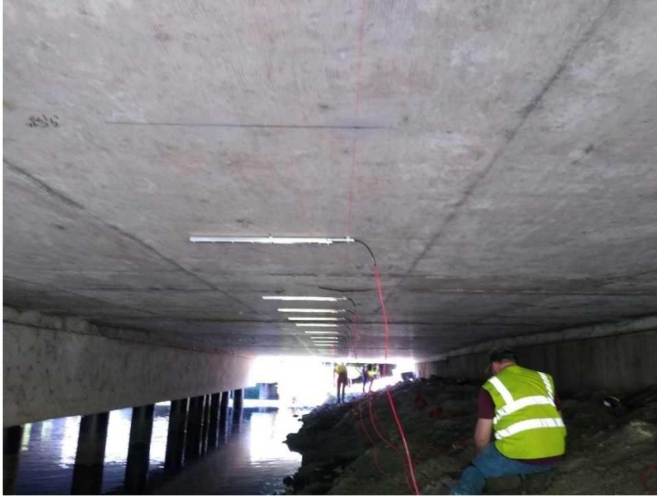
Figure H.1: Strain gauges installed on the West span of Bridge 27925.
