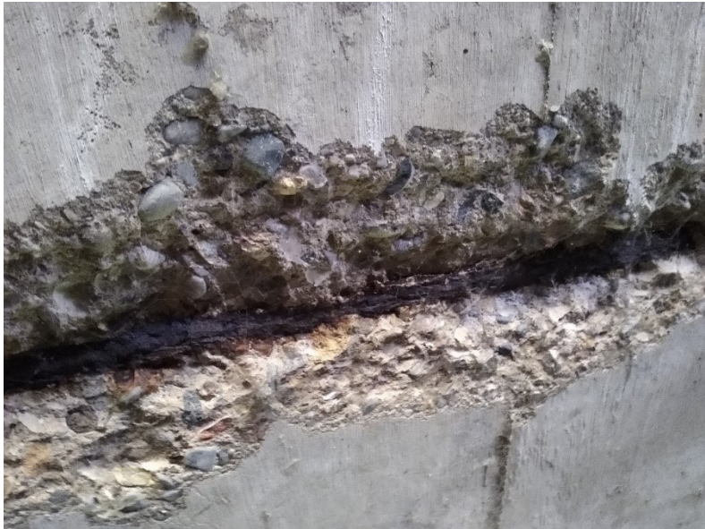
Figure A.16: Exposed steel reinforcement in Bridge 27925.
