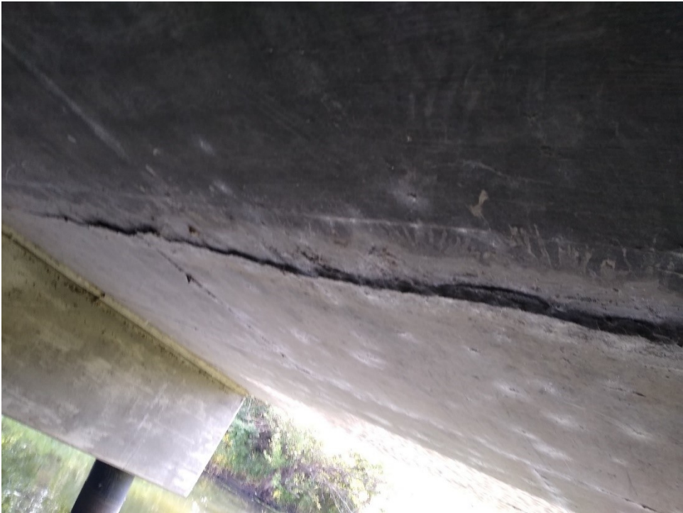
Figure A.10: Cracking observed in Bridge 27909.
