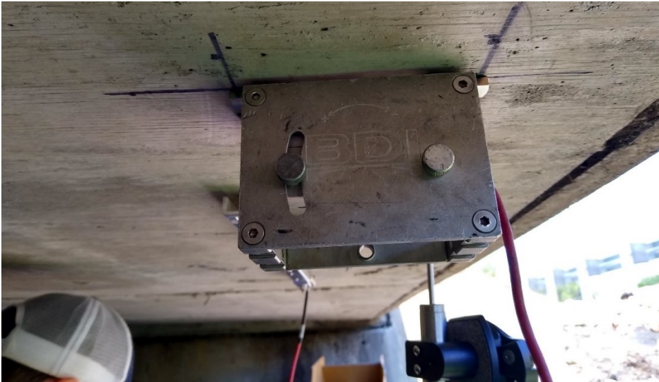
Figure F.2: Tiltmeter installed perpendicular to traffic direction on the North side of Bridge 27926.
