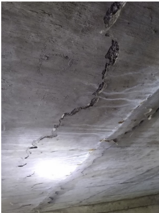
Figure A.8: Cracking and spalling observed in Bridge 27926.
