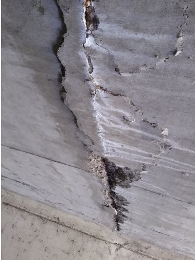
Figure A.15: Crack and spalling observed in Bridge 27925.
