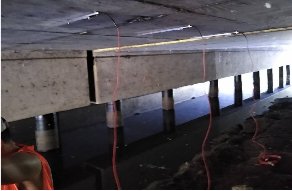
Figure F.1: Strain gauges installed at midspan of the West span Bridge 27926.
