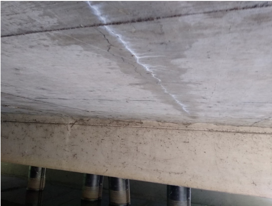
Figure A.14: Crack observed in Bridge 27925.
