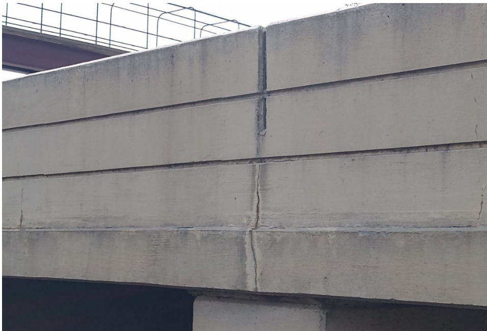
Figure A.12: Deflection joint and barrier crack in Bridge 27926.
