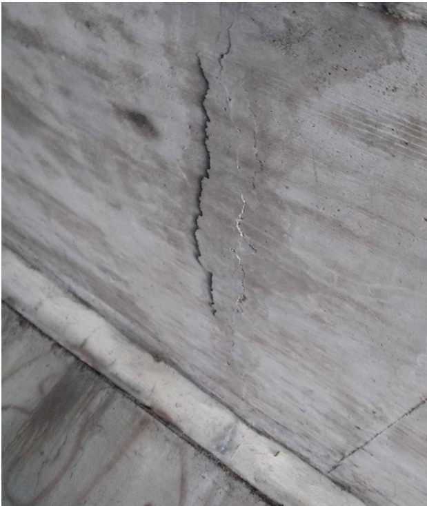
Figure A.6: Cracking and spalling observed in the slab of Bridge 27909.
