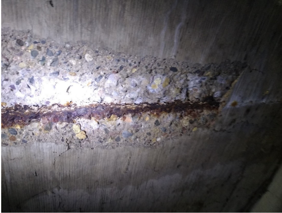
Figure A.7: Exposed steel reinforcement observed in Bridge 27909.
