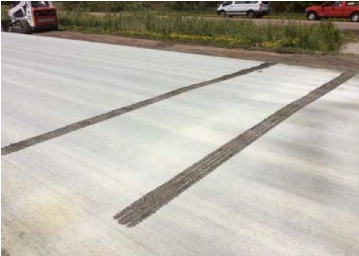
Figure 2.5 Damage in Cell 624 due to early loading
