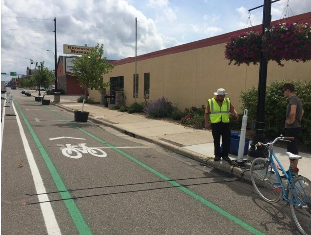
Figure 5.1 Installation of an automated bicycle counter in Alexandria
