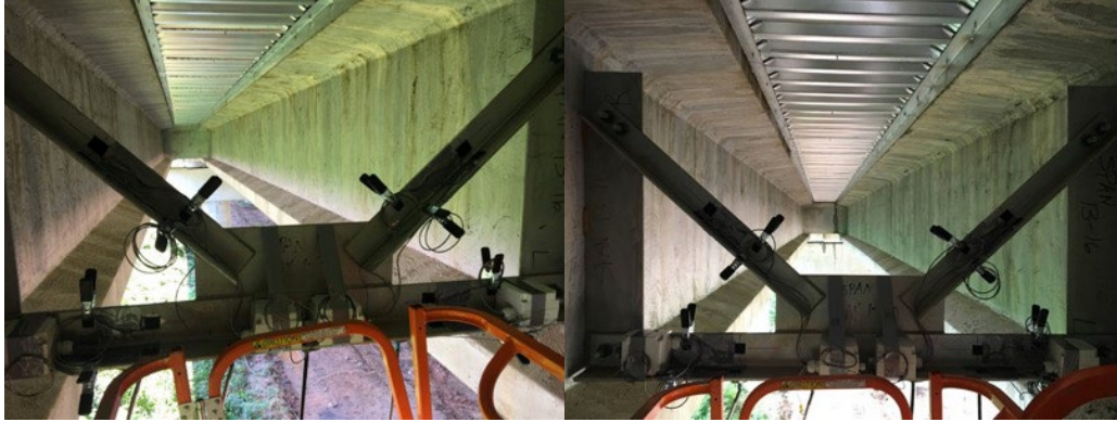
Figure 59. Photo. Final product of strain gauges installation and connection to wireless sensing units for Bay 1 (left) and Bay 3 (right)
