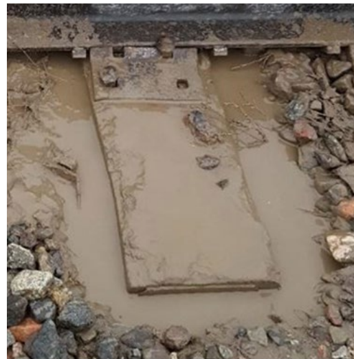
Figure 2. Photograph of mud pumping from no maintenance situation
