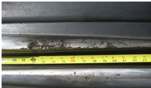
Figure 1. Surface damage on the wing rail
