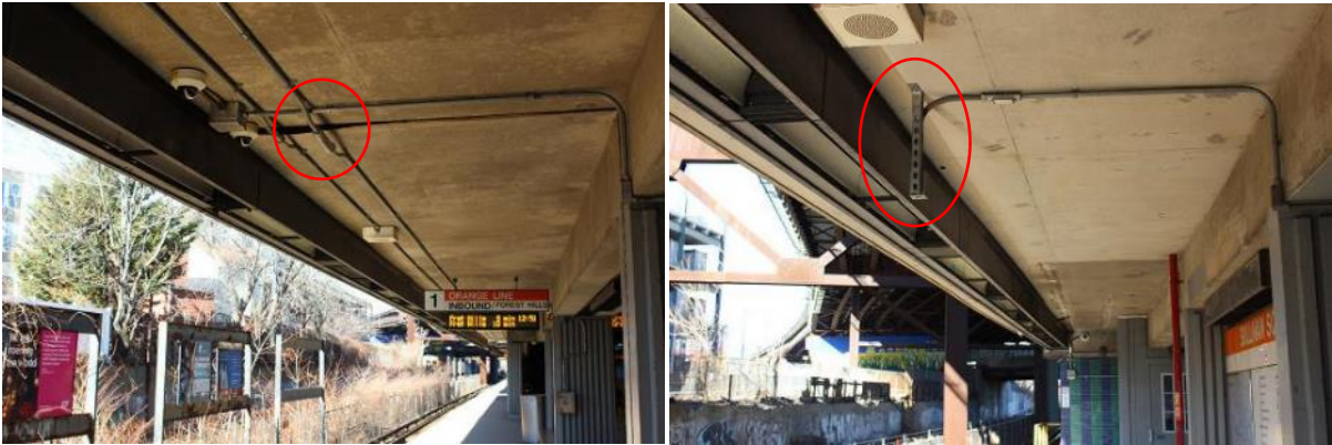
Figure 2.11: Placement of wireless device detectors at Sullivan Square
