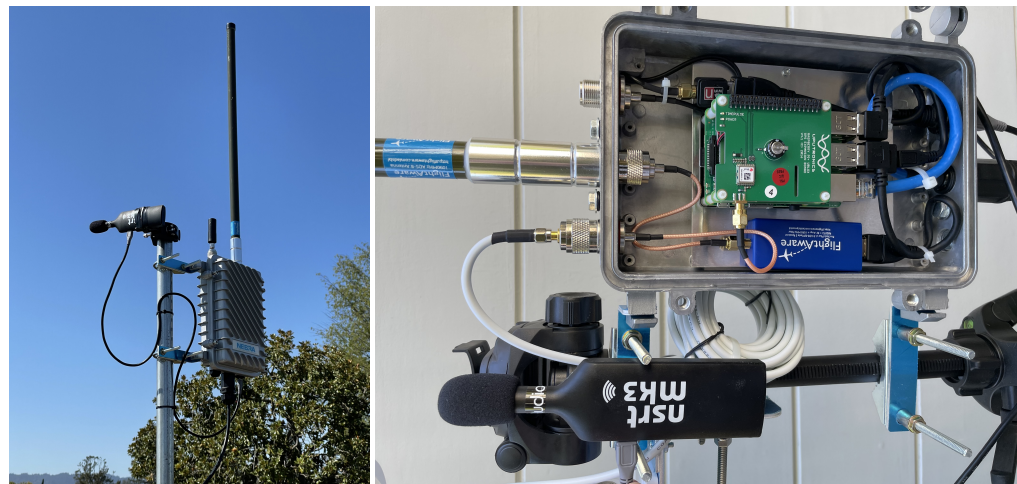
Figure 1. Sensor controller rooftop deployment with ADS-B and SLM (left), Sensor controller components (right).
